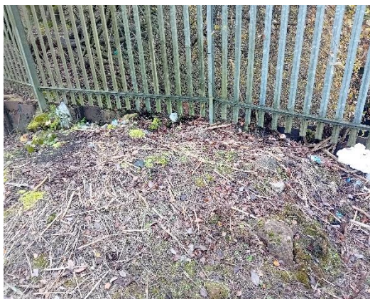
Photo 5: Himalayan balsam and Japanese knotweed growing adjacent sheet piling in raised area
