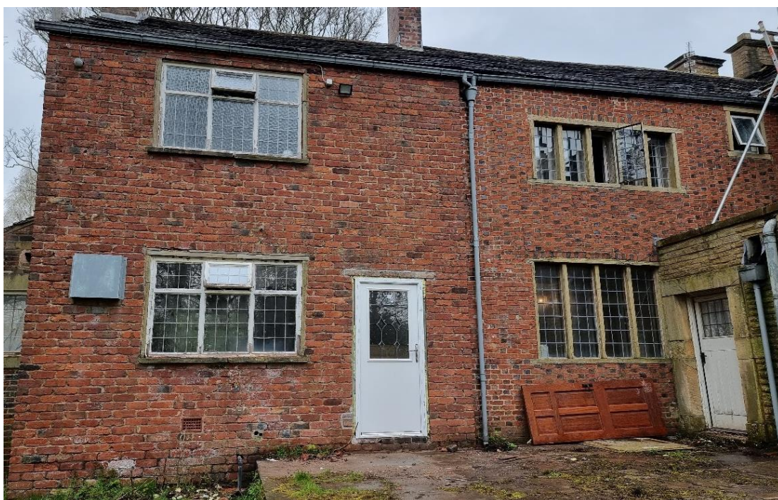
Fig.11: The west elevation of the brick wing shows evidence of reconstruction works as the left half is laid in stretcher bond and has vent bricks. This could suggest either the wall has been rebuilt indicating a cavity wall or this section of the elevation has been refaced and the original brick work has remained in situ. The windows to this refaced section are modern.
