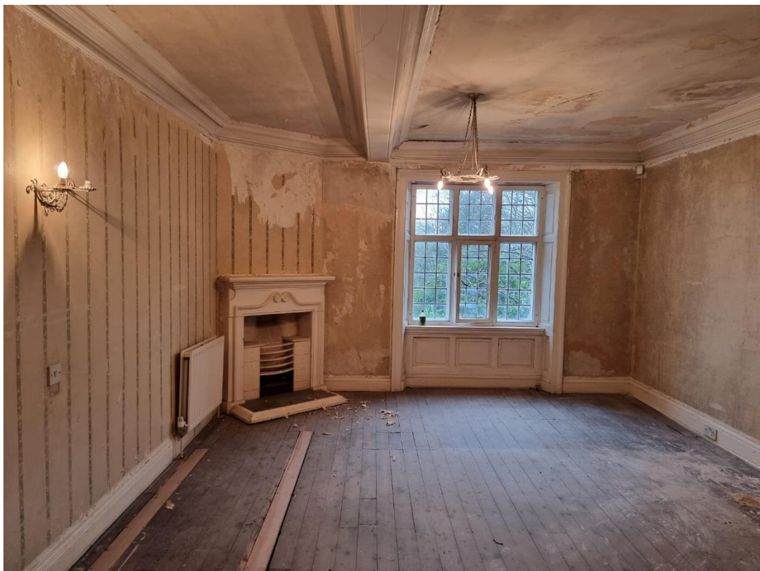
Fig.31: Bedroom 1, to be replastered with lime.
