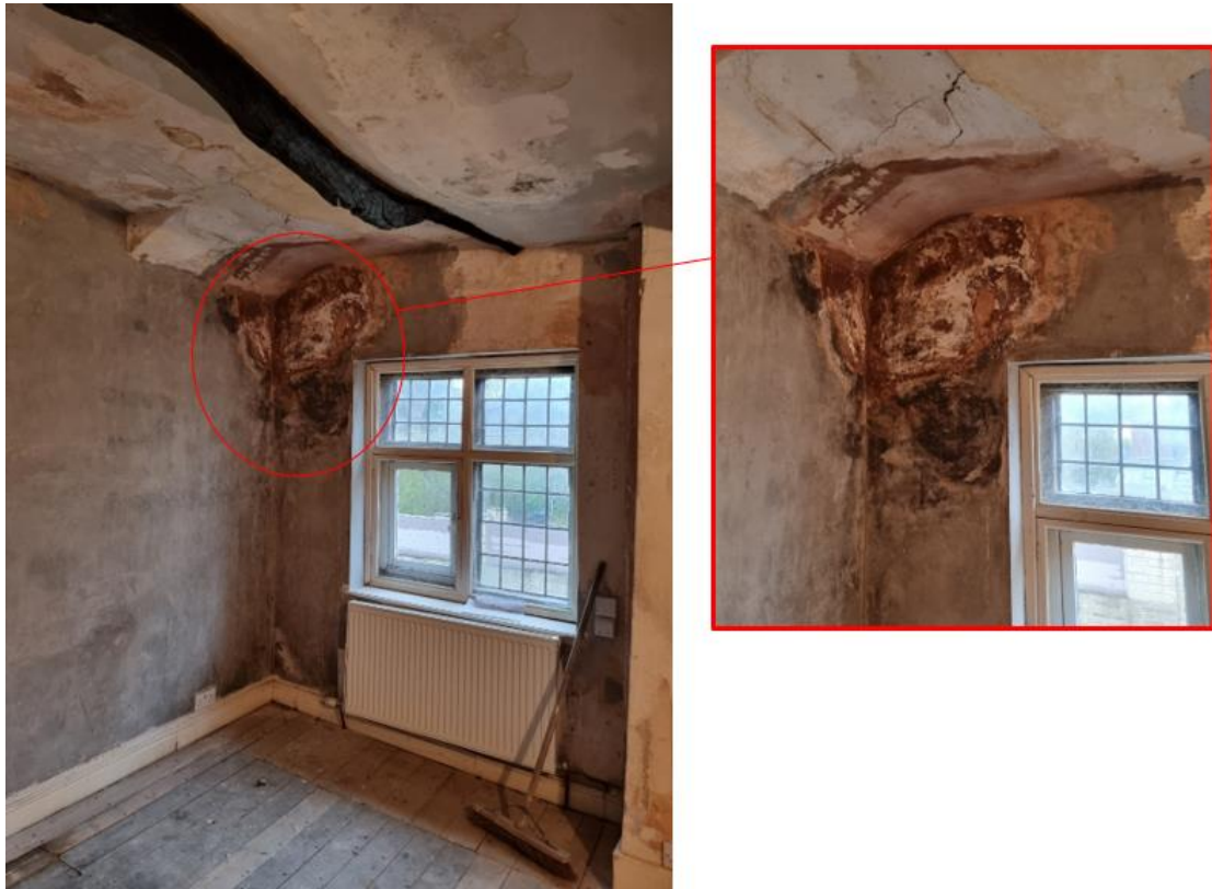
Fig.34: Red circle denotes an area of gypsum plaster to be removed following water ingress. The area is to be allowed to fully dry out before lime plastering.
