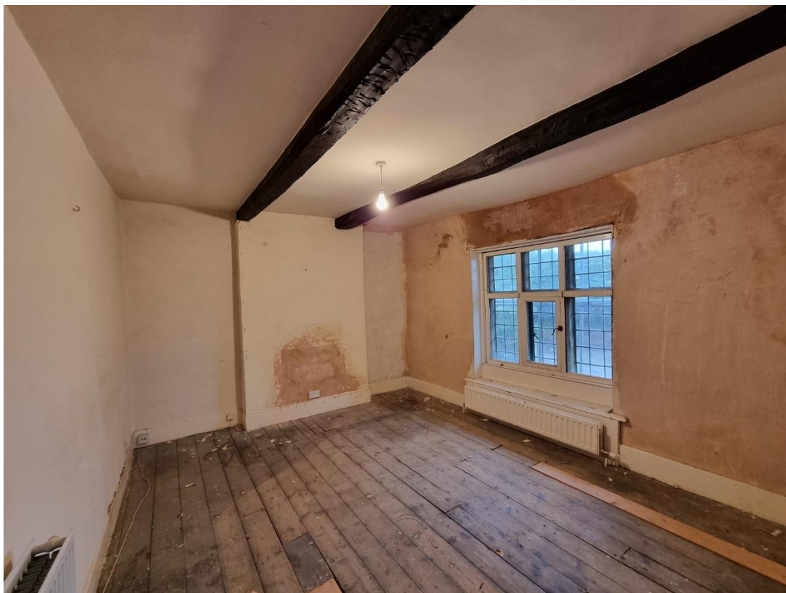
Fig.36: The gypsum plaster above the window is to be allowed to fully dry out before replastering with lime.
