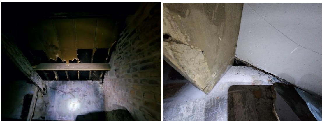
Photographs 15 and 16 showing the interior of the roof space showing wooden cladding and crack in brickwork, respectively.
