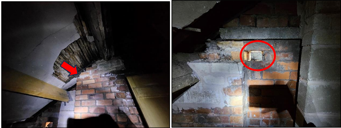
Photographs 11 (left) and 12 (right) showing gaps along gable end and hole in brickwork, respectively.
