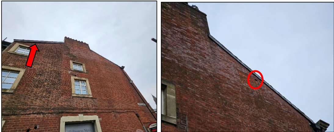
Photographs 2 (left) and 3 (right) showing gaps under barge board and hole in brickwork, respectively.
