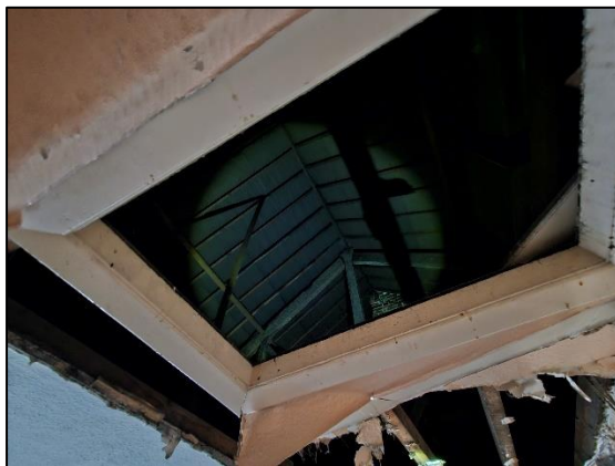
Photograph 20 showing broken ceiling giving access to the loft.
