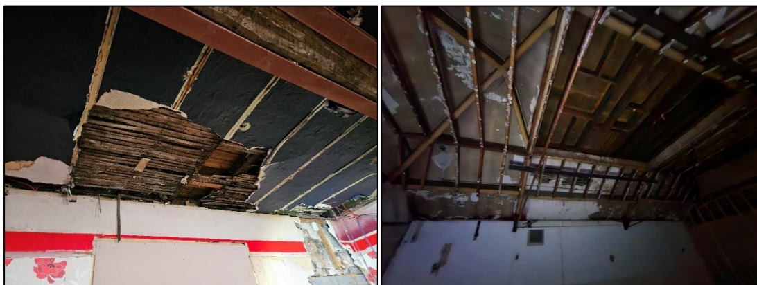
Photographs 21(left) and 22 (right) showing PRFs at the first floor.
