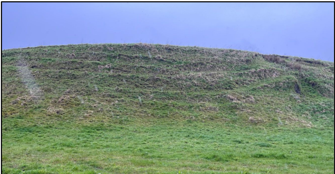
Photograph 2.1: Near-surface instability observed during site visit.
