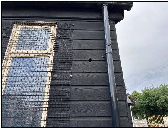
Figure 6: Holes in the wood cladding.
