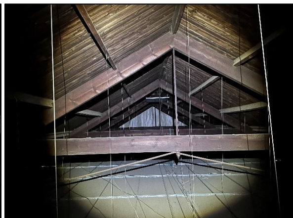
Figure 13: The void over the suspended ceiling.
