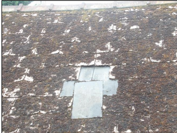
Figure 10: Slipped tiles on the roof of the building.
