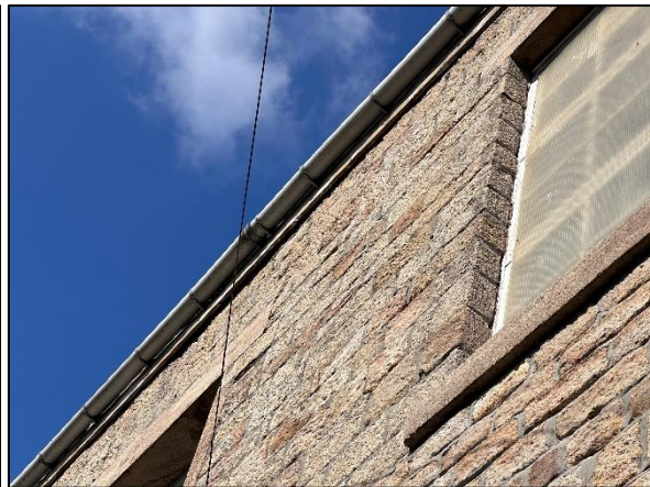
Figure 11: Voids behind the fascia boards.
