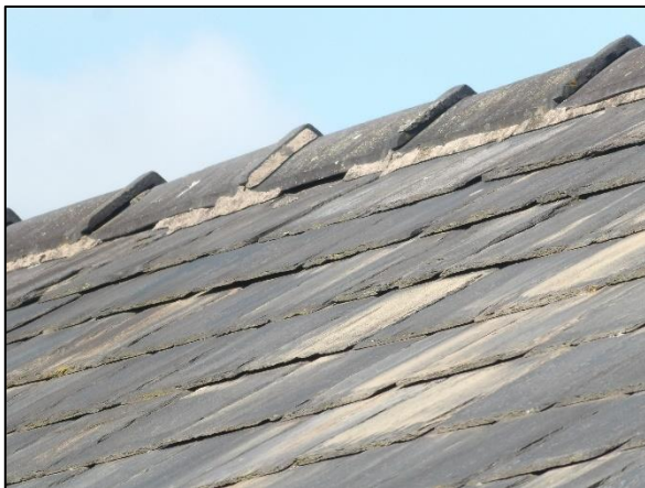
Figure 12: Voids under the ridge tiles.
