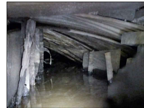
Photo 3: Steel drooping into culvert under shed (Hopwood House)
