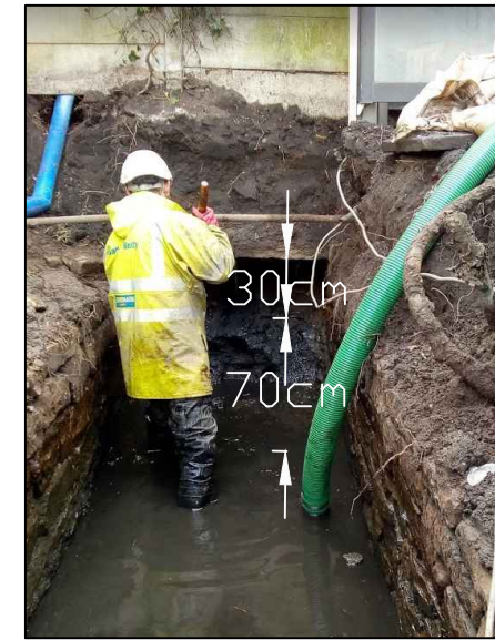
Photo 1: of silt looking towards Hopwood House. 70cm deep silt & 30cm freeboard (clear)
