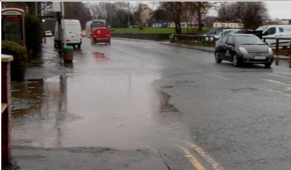
Photo 1. Highway flooding that used to occur regularly before the major works to desilt the culvert under Thornham Rd was undertaken by the Council Highways team. This could easily recur because the culvert in Hopwood Farm house land has not be adequately desilted and is not very accessible for desilt activities.
