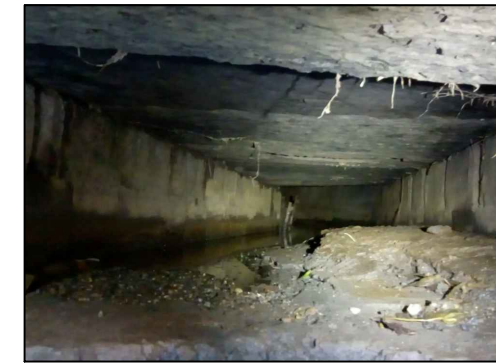
Photo 2:- Deep layer of silt still in culvert under Hopwood House 'garden' (April 2019).
