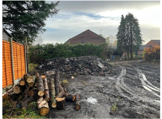
Photo 2: Large pile of soil and log pile located at the north eastern boundary of site.
