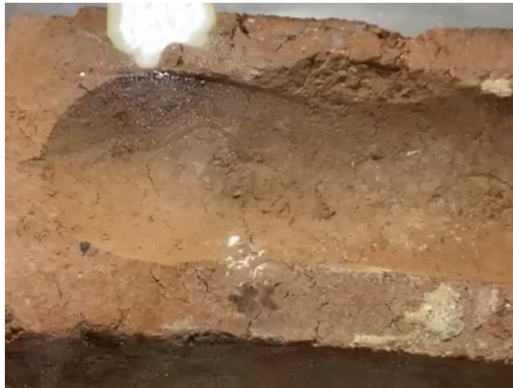
Fig 1: Representative brick sample taken from Brunswick Street – December 23 – Uneven appearance and failed Water absorption test
