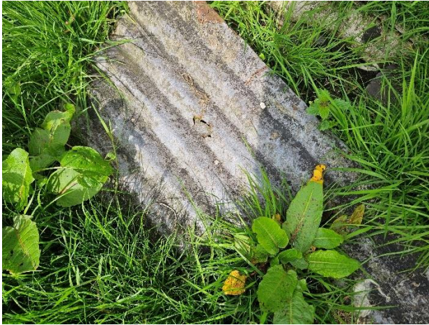
Figure 2.3: Potential Asbestos (including asbestos cement) noted along the northern boundary.
