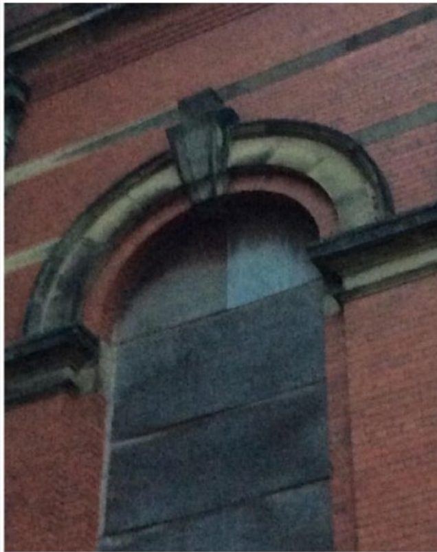
Figure 1: Location of bat roost entry point identified at the base of the keystone over a boarded up
