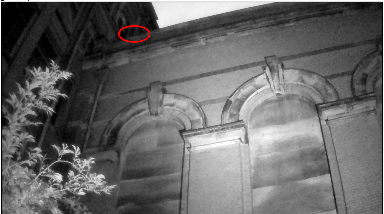
Photo 07. Location of crack near roof common pipistrelle emerged from on 19.09.2023 (viewed from ground)
