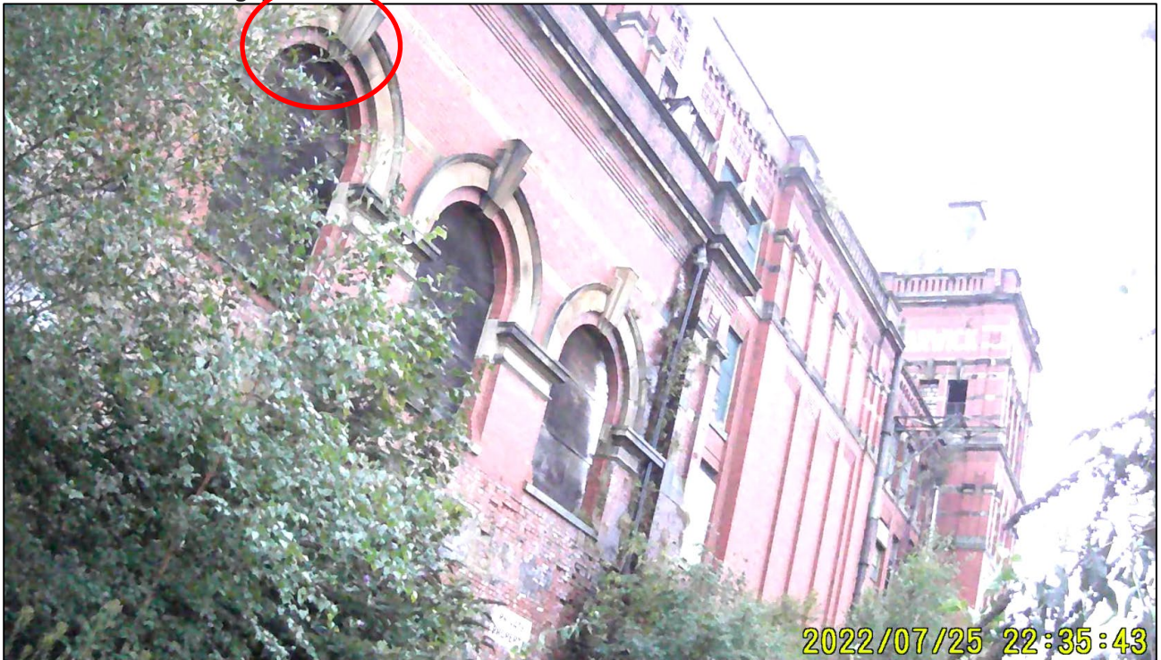
Photo 06. Potential emergence from top of window board on eastern elevation 31.08.2023 (time and date incorrect in image)
