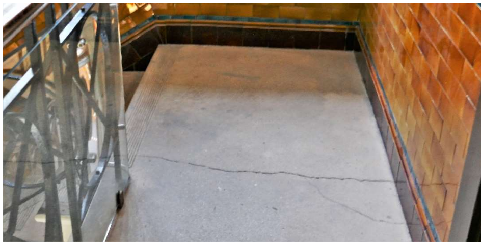
STR6- There is a crack in the landing of the stairway directly above the entrance area. It is not clear if this is new or progressive but would warrant further structural investigation and monitoring
