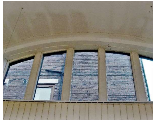
D16- Condensation staining to the ribbed ceiling structure of the library. A boarded lining to the window reveal and impervious finishes has led to spalling..
