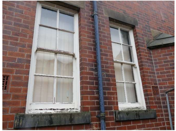
W6- The sash windows show signs of rot within the cills and bottom rails where decoration and seals have failed. Some cutting out and replacement will be required.
