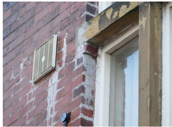
ST12- Salt staining to the end gable of the upper meeting room may be from a high salt content in mortar used for re-pointing. This will need to be removed and possible raked out and replaced to address the issue.
