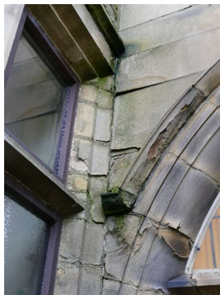
ST5- Spalling of the facing following saturation from run off from the roof abutment with the old town hall above.
