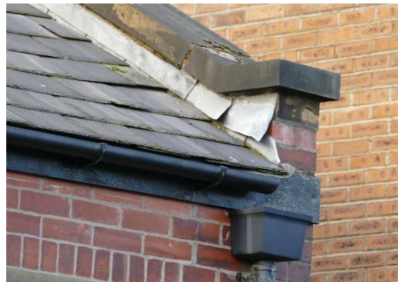
R16- Flashings to the coping of the east corner of the lower library roof have lifted and require to be re-dressed and clipped. The coping joints are open and should be re-pointed and the gutter outlet and dropper into the hopper are missing.
