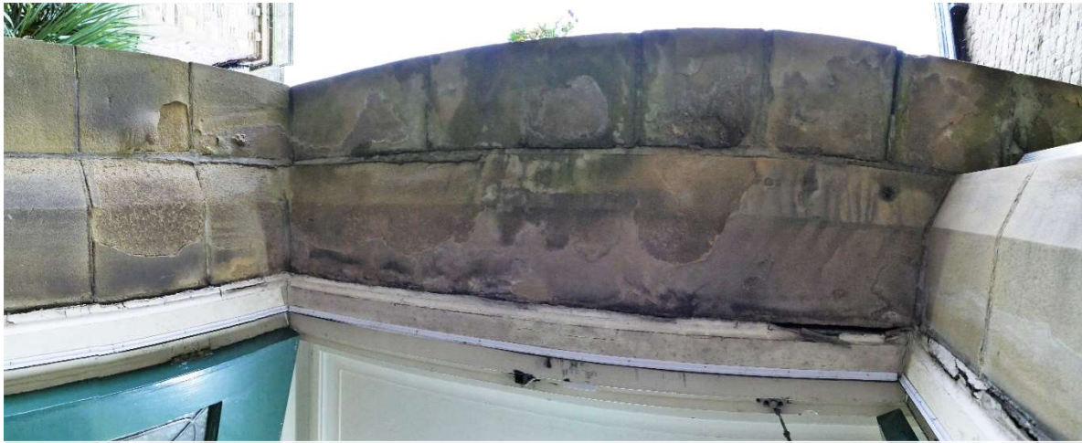
STR5- The external facing of the stone panel over the entrance bows out from the internal structure. This is exaggerated in the photograph above by the wide-angle lens but can be seen in the variation in the width of the joint. The gap has been pointed in the past but has some new hairline cracking.
