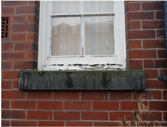
W7- The sashes are seated on stone cills and open joints around the frame have allowed water to lodge in the timber.
