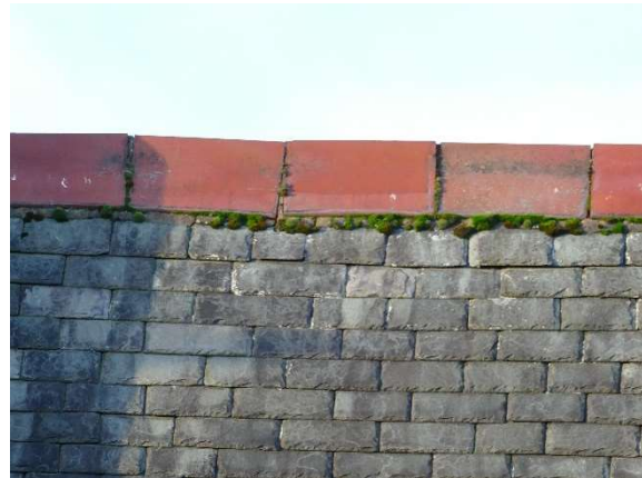
R8- The line of the ridge is uneven and some levelling is required in the bedding when it is replaced and the tiles re-pointed.
