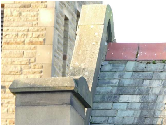
ST9- Open joints and a displaced capping stone to the coping above the front entrance.
