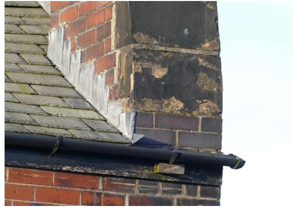
R12- There is no outlet to the gutter of the roof over the meeting room and this washes over in heavy rain.
