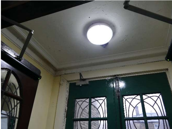
D1- Spalling paint to the ceiling of the porch is likely to be from successive overpainting curling the paint below or from incompatible paint finishes. Re-decoration is required.
