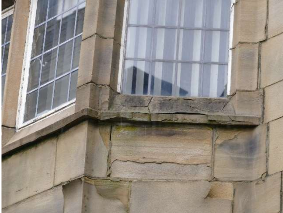
ST7- The stonework to this cill has spalled and fractured and requires an indent repair or replacement once the movement has been arrested.
