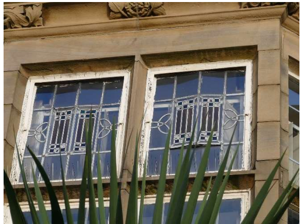
W2- Leaded glass panels to the upper front oriel window have buckled and require careful specialist conservation and re-leading. The swivel hopper vents also require repair.
