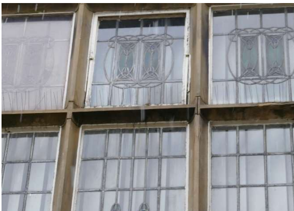
W3- Leaded lights over the main entrance retain their original glass and leading. Comes are oxidised and some welds split and conservative specialist repair is now required. The left hand panel has five broken quarries. In-situ repair might limit the loss of historic glass. The sealed protective sheet should be replaced with polycarbonate with a ventilated perimeter and non ferrous fixings.
