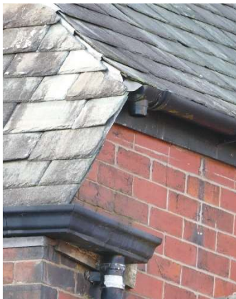
RWP3- The gutter to the back of the stairwell has no fall pipe and expels onto the roof below.
