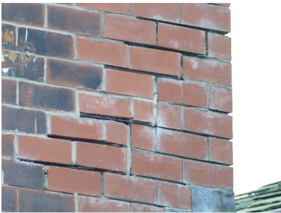
STR7- Brickwork to the west corner of the library appears to have become vertically displaced along the line of a step dpc. This corner was re-built as part of the 2002 refurbishment. The upper brickwork appears to be corbelled off the existing while the lower section has settled/rotated.
