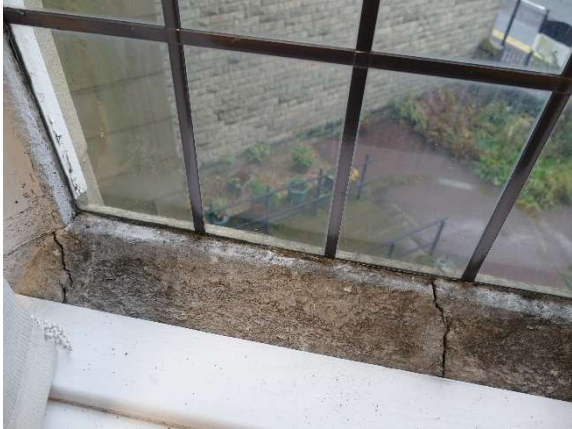
D11- The movement within the oriel window is exhibited in fractures in the stone cill and to the external head.
