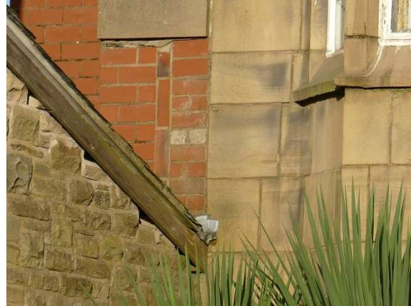
R6- The abutment of the old town hall roof to the library has a very shallow upstand and an open end. Overflow from this detail has significantly damaged the stonework below, to the front of the library.
