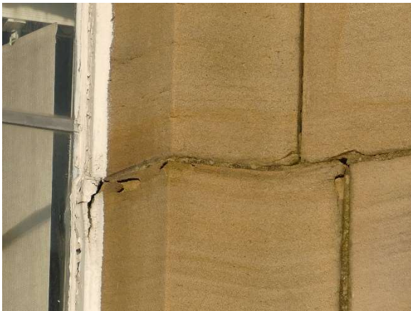
W1- The displacement of the stone to the side of the front oriel window has caused it to split and spall. This has not fractured the glass yet but is allowing moisture to penetrate around the lead glass panel.
