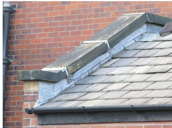
R14- The flashings to this coping, to the lower library roof, are not clipped and may be loose where they dress under the copings. Closer inspection is required.
