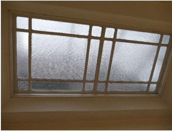
W5- laylights below the library skylight are timber framed with textured glass panels to a geometric design. These appear to be in reasonable condition but consideration could be given to installing safety film to prevent shards falling if they break.
