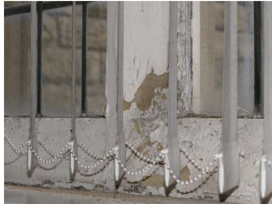
D12- Glass paint forms a barrier to the evaporation of moisture in the stonework and should be removed completely.
