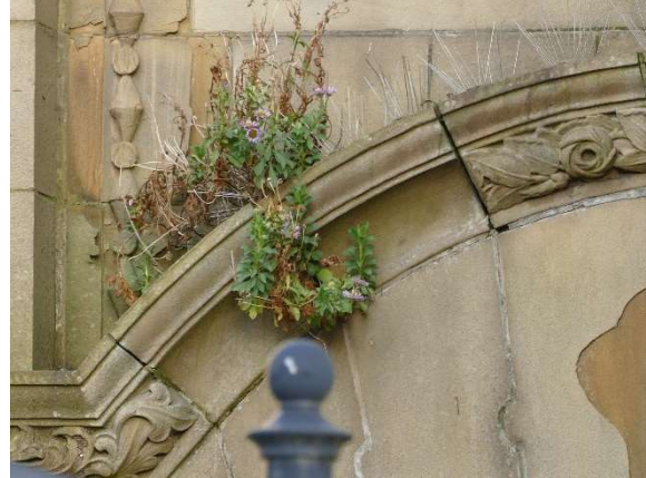
ST8- Open joints in the label mould over the entrance have led to vegetation taking hold. This should be removed and the joints fully re-pointed.
