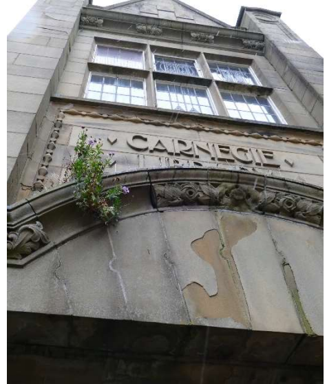
ST3- Spalling of face bedded stone over the doorway and vegetation in the open joints of the label moulding. Loose spall should be removed and the stone re-dressed and pointed in lime mortar.
