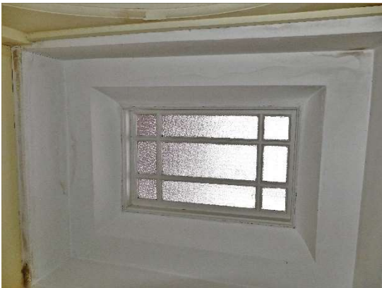
D15- The sides of the laylight that abut the continuing walls above show signs of staining where water has penetrated the flashings or over run the drip tray above. Condensation may also be forming on the underside of the uninsulated flashings.
