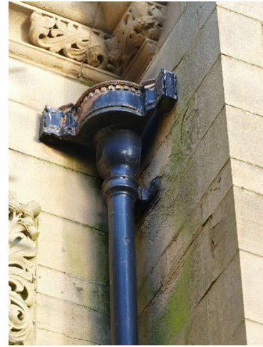
RWP2- The cast iron hopper to the head is corroded and requires de-rusting and re-decoration..
