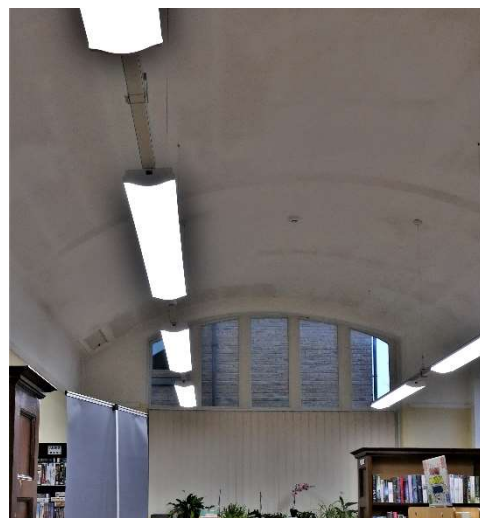
D4- There is widespread condensation staining to the barrel vault ceiling of the lower library. Improved insulation, along with an assessment of condensation risk, would help to reduce this in future but re-decoration is now required.
