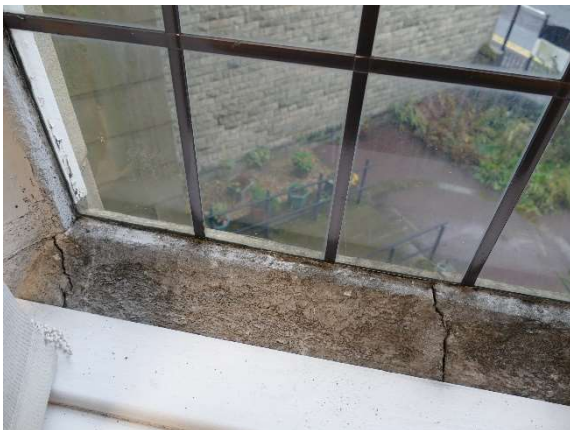
STR3- The displacement of the bay has sheared the cill of the side light in two places and the other in one along with a split in the head.
