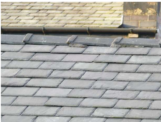
R15- The bedding to the concrete ridge tiles of the lower library roof require re-bedding and pointing.
