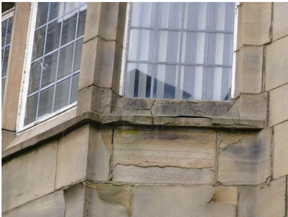
STR1- The oriel window cill is split and the surrounding masonry displaced suggesting structural movement.
