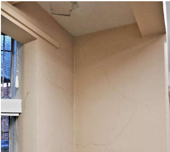
D3. Spalling paint to the ceiling of the oriel window bay may be from incompatible paint finishes or successive overpainting. Access into the void above would identify if there is a water ingress issue. Cracking on the side wall could be drying out cracking of the plaster or may relate to movement visible on the external wall.
