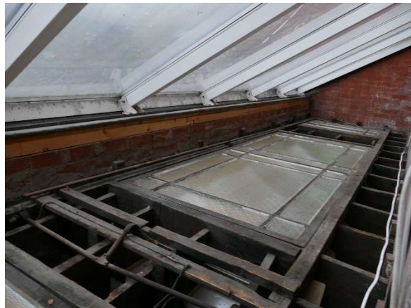
SK2- The dried timber frame spans between the beamed structure of the library and supports the timber laylights. Putty to the lay lights has cracked and spalled and consideration should be given to removing the putty and installing safety film before re-puttying the textured glass panels.
