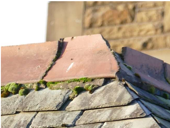
R13 The ridge detail to the corner of the roof is weathered and uneven and will not be protecting the head of the mitred hip flashings.
