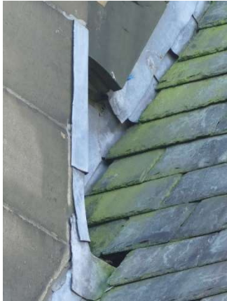
R17- Where the abutment detail of the entrance gable dresses around the rear piers the upstand and laps appear to be minimal and may be being inundated in heavy rainfall conditions.
