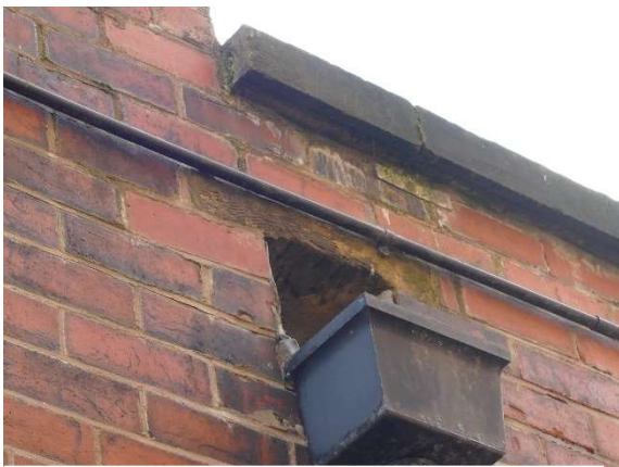
ST11- Open joints in the coping require re-pointing. The outlet chute requires re-dressing to protect the timber liner.
