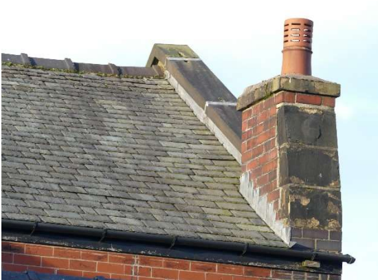
R9- A chimney to the east corner of the library exhibits a number of issues that may be contributing to moisture staining in the ceiling below
