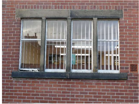
W8- The windows to the library east side are fixed and exhibit the same deterioration of the cill and some open joints to the transom.
