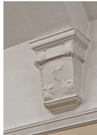
D14- Successive overcoating of paint has concealed the detail of the corbels in the meeting room and have led to the paint curling and spalling. Careful removal will uncover the original detailing.
