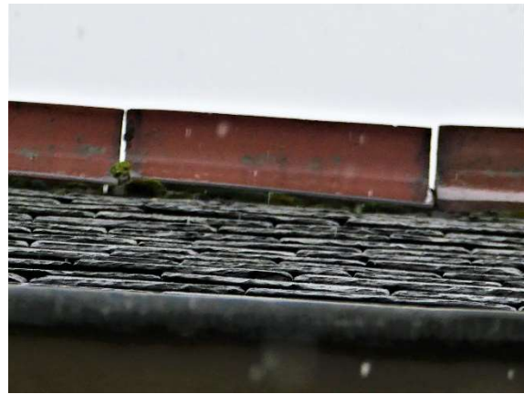
R20- There are significant gaps between the red clay ridge tiles and some could soon be displaced in windy conditions.
