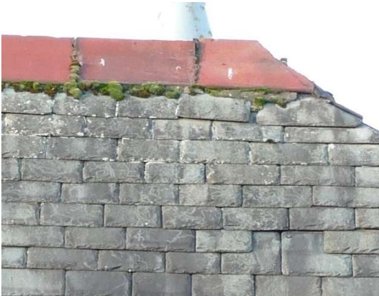
R7- The joints and bedding of the ridge tiles have weathered and they are now allow in need of re-pointing and bedding. A slate is missing below this section.
