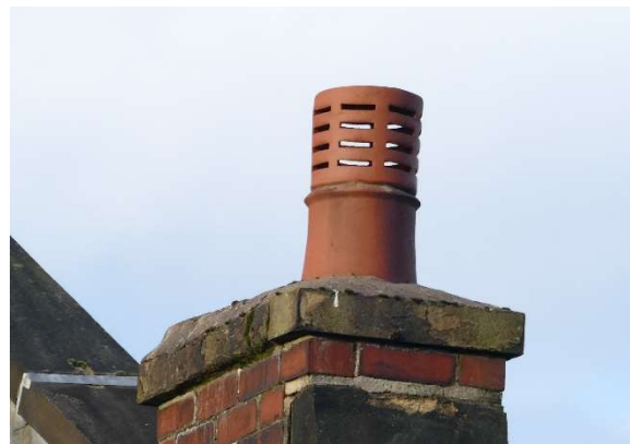
R10- The flaunching to the chimney is split and lifting and the pot appears to have a slight lean. Open joints may be allowing water ingress. There is also a significant gap between the brickwork and the stone slabs that face the east face.
