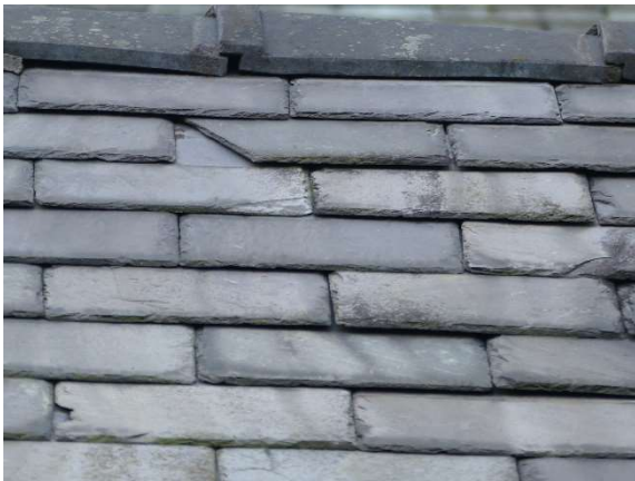
R19- The slate is showing signs of spalling and of splitting and those most compromised will need to be replaced to extend the life of the roof.
