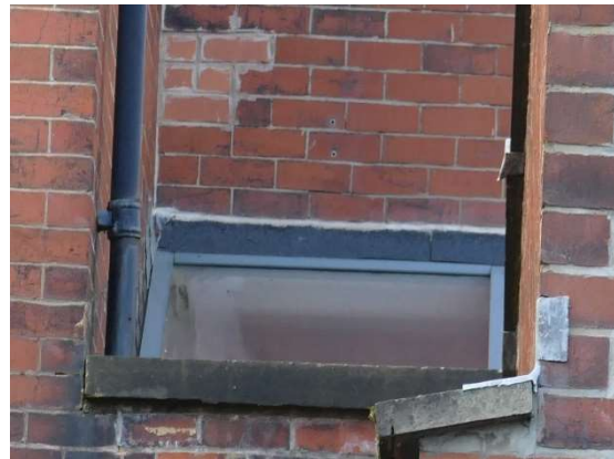
SK4- Where visible from ground level, the top flashing of the skylight can be seen to be a felt or artificial flashing. Cover flashings to the end profile can also be seen to be missing. This and condensation are likely to be possible sources of water ingress.
