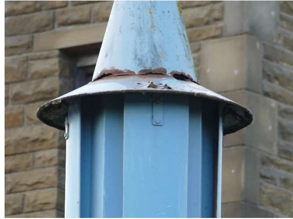
R18- When viewed from the back of the library, the ventilation turret can be seen to be heavily compromised by the corrosion. This will be allowing water into the ductwork below
