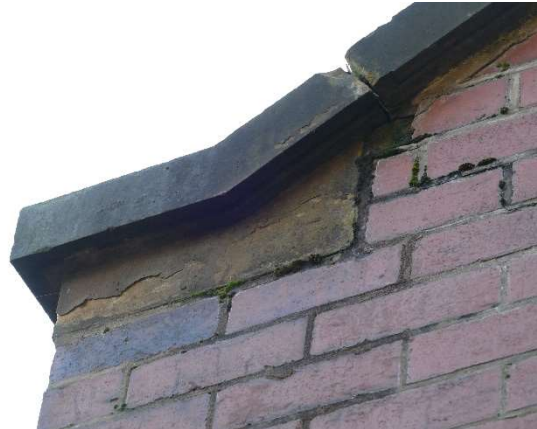
ST10- An open joint to the kneeler on the east corner of the library has allowed moisture to penetrate and mould to take hold. Moisture will penetrate to the interior of the building if this is not addressed..
