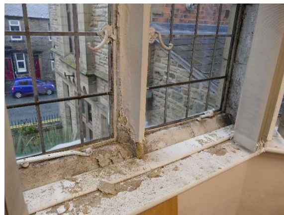
W9- Saturation of the window stonework, through open joints and exposure has led to extensive deterioration in the matrix of the stone and to spalling as seen here in the oriel window to the upper reception/meeting room. Corroding dowels are also likely to have contributed
