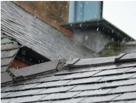
R21- Open joints are also visible in the line of the grey ridge tiles to the lower library wing.
