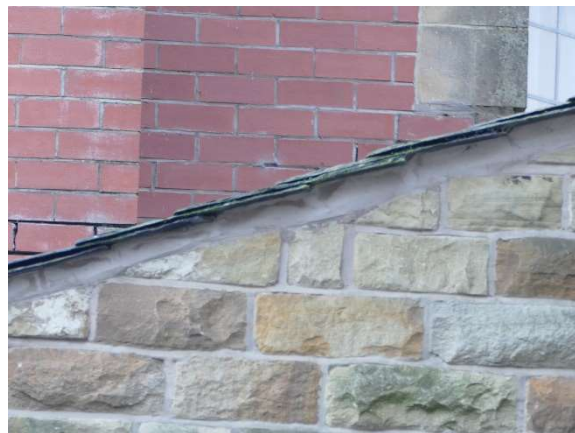
STR8- There is also a stepped joint visible in the west side of the stage area. This is only just visible from ground level and would warrant closer inspection.
