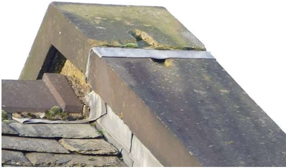
R11- Copings to the library are set on lead flashings and these are dressed over the joints. Recesses for cramps are open and likely hold water
