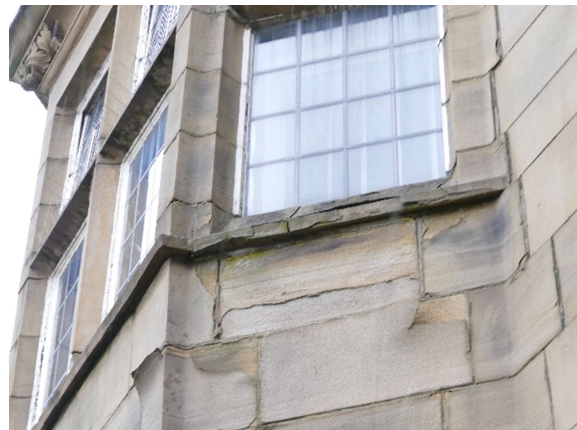
STR4- There is a visible bow in the line of the lower cill of the oriel window and a fracture line where it has started to pull away from the face of the adjacent walling.
