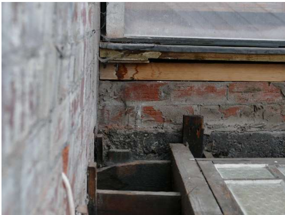
SK1- Staining is visible to the wall plate and may be run off from the end of the condensation tray above or from past water ingress at the head of the skylight.
