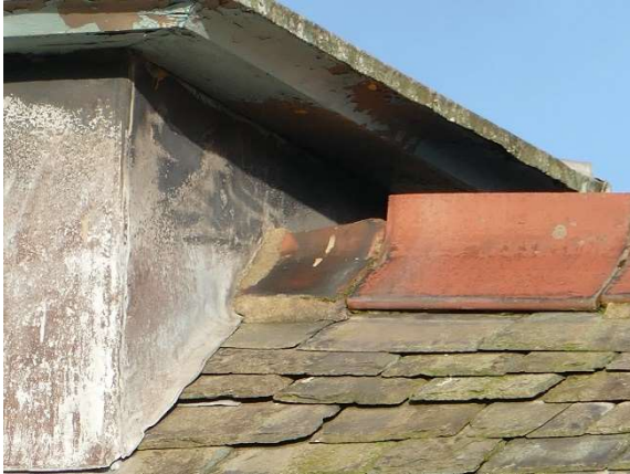
R5- The corner seam of the turret base cladding appears to have opened at the top. Red clay ridge tiles have open joints.
