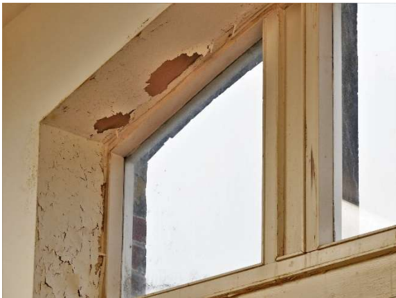
D13 The surrounds to the rear arch headed windows has been re-plastered in gypsum plaster and painted with vinyl paint. Moisture in the fabric has been trapped leading to spalling.
