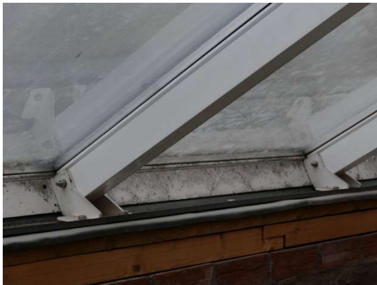
SK3. The frame and glazing of the skylight and the laylights below all require to be cleaned. It is not clear if the drip tray around the perimeter has outlets or is sealed..
