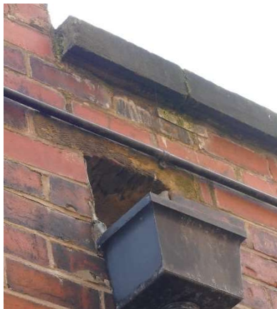
RWP4- Staining from open coping joints and exposed timber liner to the spitter. Pointing of the coping and re-dressing of the lead spitter tray are required.
