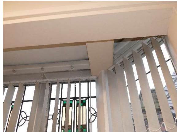
STR2- The head of the oriel window has been reinforced with steel in the past but the lower section appears to have continued to rotate.
