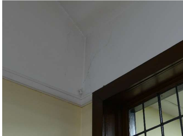
D2- Cracking to the west corner of the lower library maybe from movement of the roof structure above or from moisture behind the underlying plaster. There is a hipped roof and parapet gutter above.
