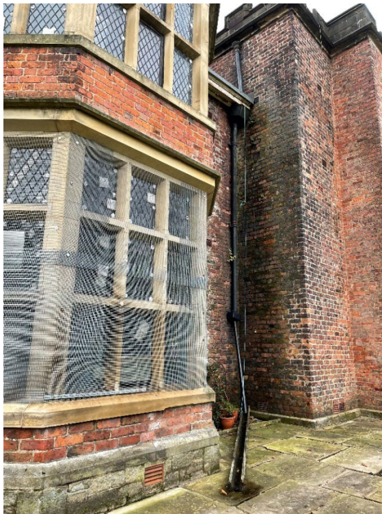
Figure 3.21 Rainwater pipe failure affecting the brickwork to the south-east of the Hall.
