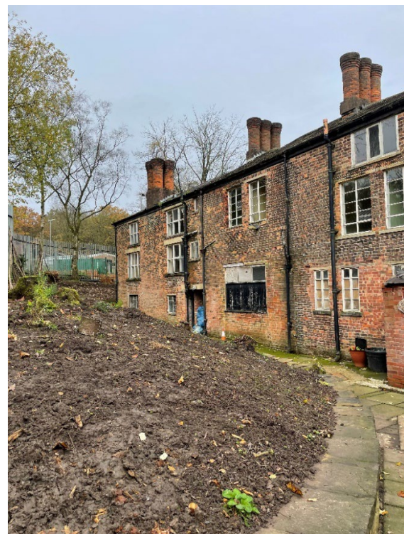
Figure 3.22 West wing of the building which is in a very unsafe condition structurally.
