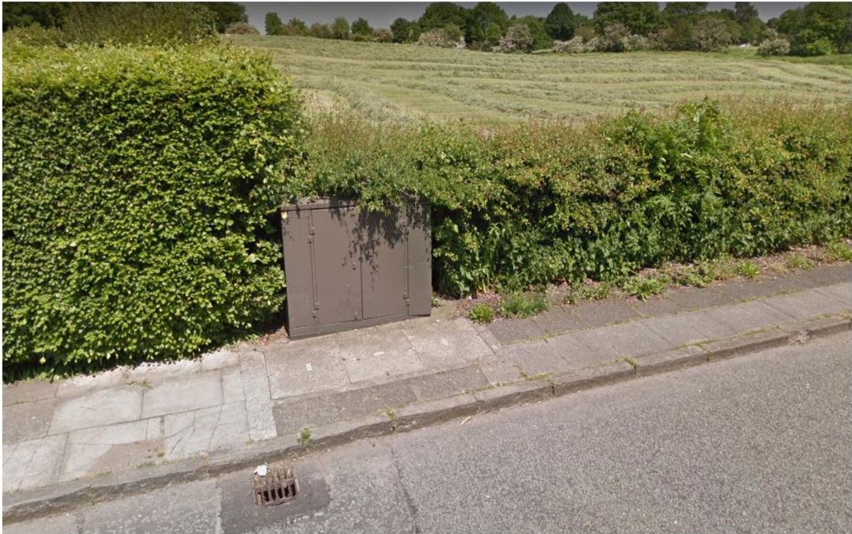
Figure 6.3 –Joint Box and Cabinet Adjoining situated on Bentley Avenue
