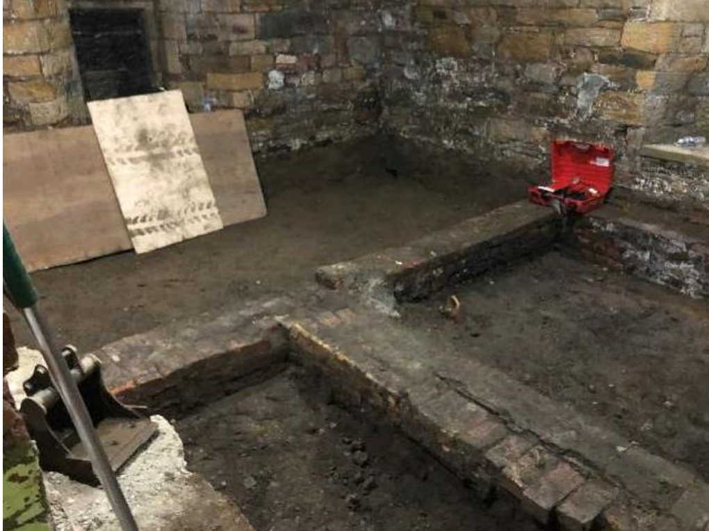
Example of below ground obstructions in B6d.
