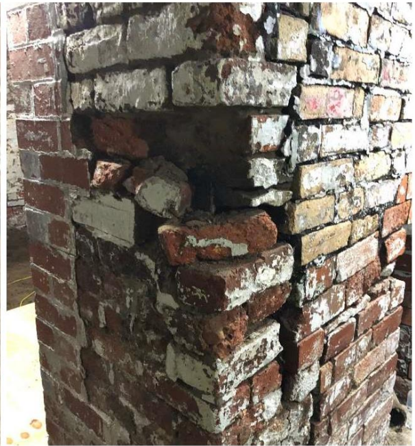
Poor condition of brickwork, not tied into fabric.
