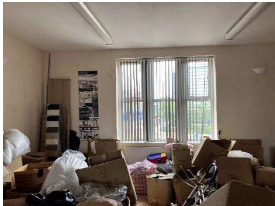
Figure 17 – View on Front Window with Minor Cracking / Staining to Top Left Corner
