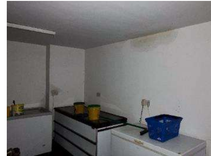
Figure 6 – Possible Damp Staining to Basement Wall
