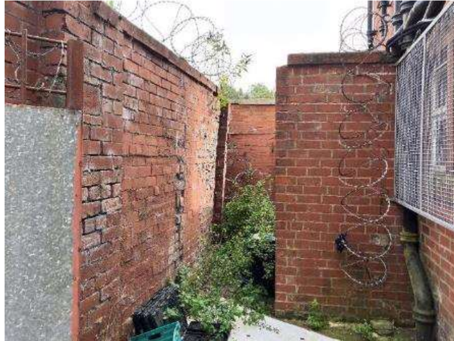
Figure 22 – View on Leaning Section of Yard Wall
