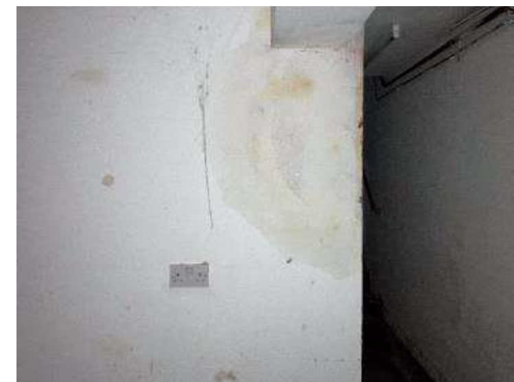
Figure 7 – Possible Damp Staining to Basement Wall
