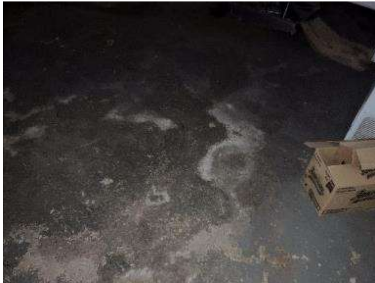
Figure 8 – Possible Damp Staining to Basement Floor
