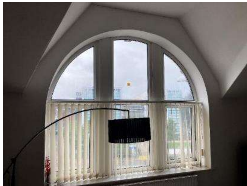
Figure 20 – Minor Cracking Above Front Dormer Between Wall and Ceiling
