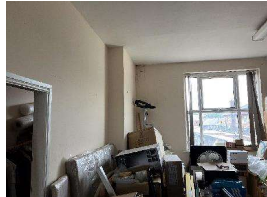
Figure 18 – View on Rear Wall with Potential Water Damage to Top Left Corner
