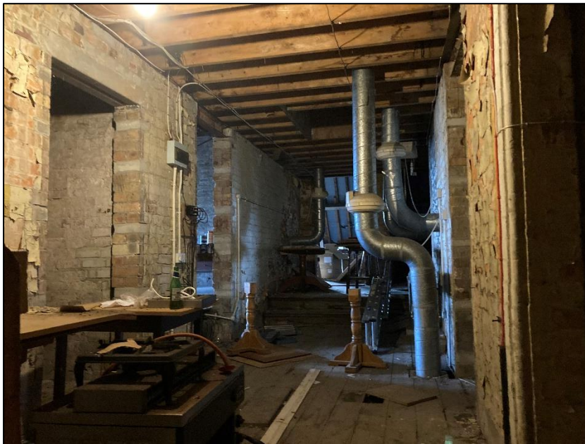
Photograph 27 showing the internal void
