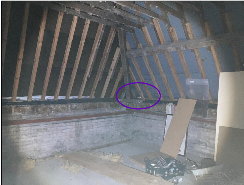
Photograph 30 showing a gap
