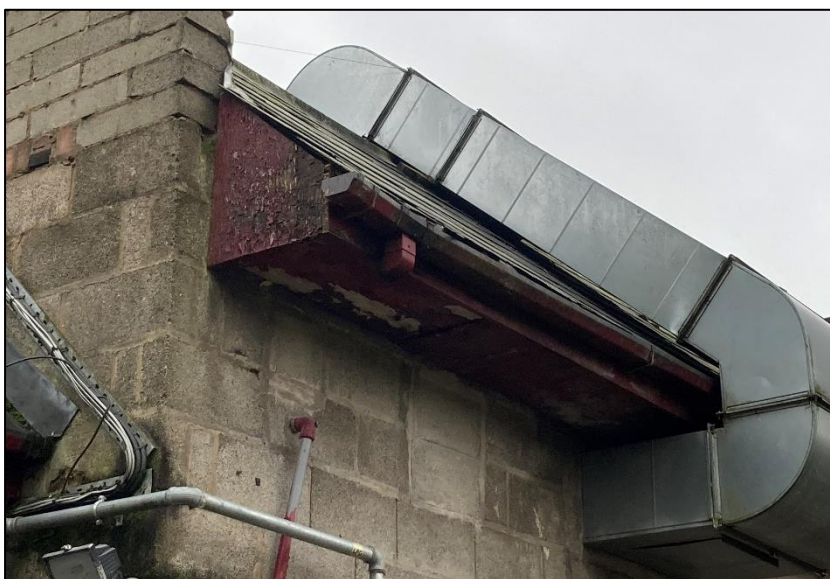
Photograph 23 showing the gaps in the soffits
