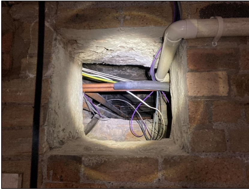
Photograph 26 showing the cavities within the walls
