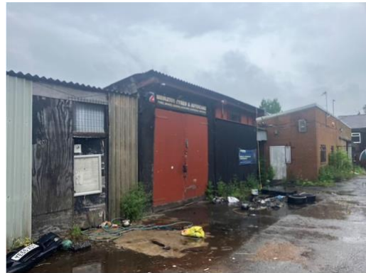
Photo 6: External view building 3. Showing poor condition and lack of insulation or hidden cavities.
