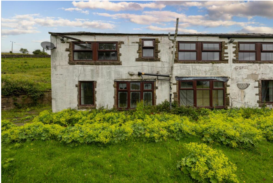
Figure 5 – View of the front elevation showing the current defects and disrepair of the property.
