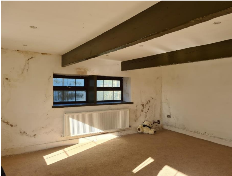
Figure 9 – View inside the dwelling showing signs of disrepair and issues with damp.
