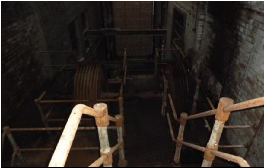
Fig 12 & Fig 13 above, Existing Rope race machinery
