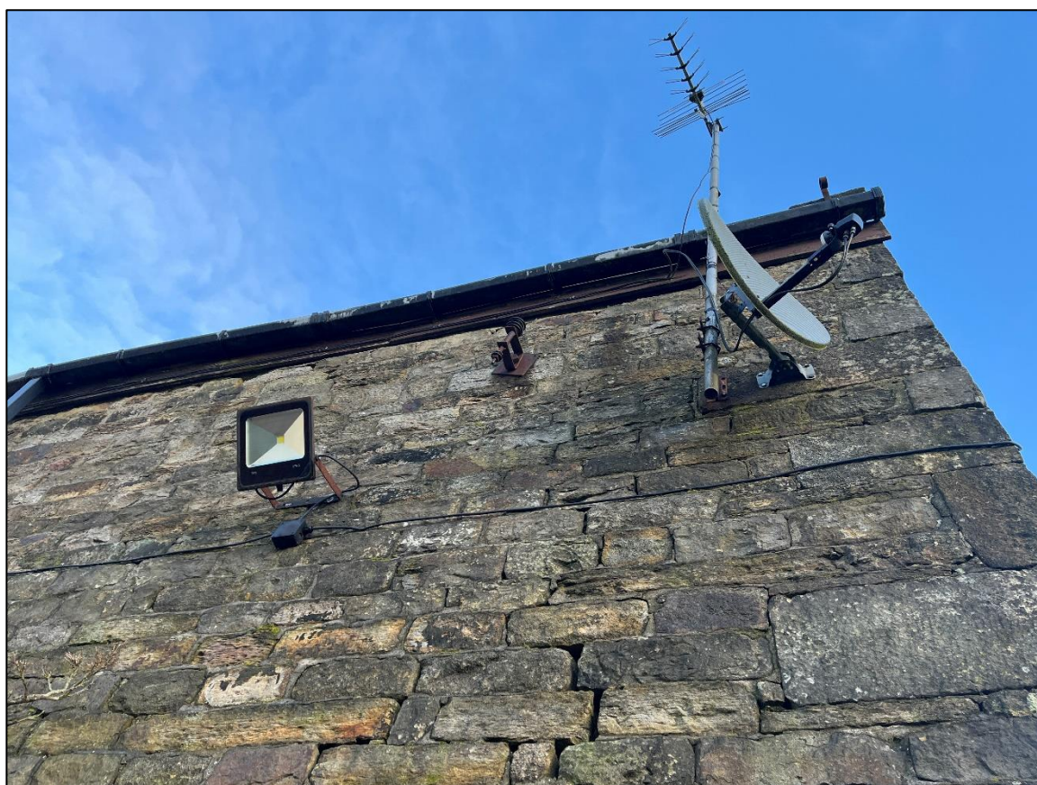
Plate 10 – Gap beneath fascia on southern aspect of B2
