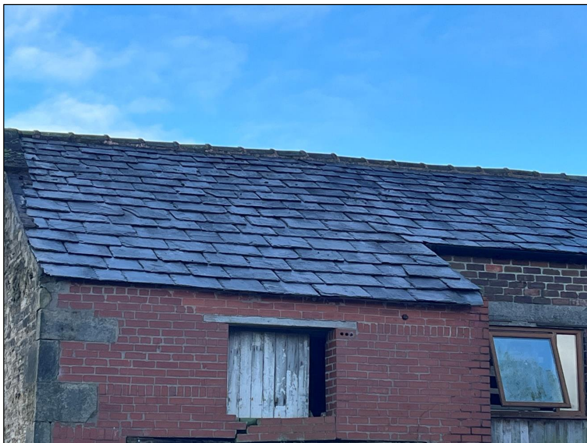
Plate 9 – Several lifted slates on northern aspect of B2
