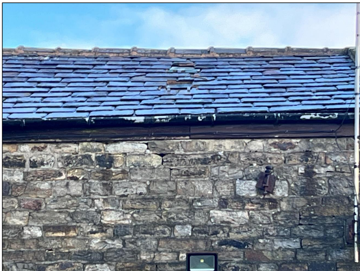
Plate 11 – Slipped and missing slates on southern aspect of B2
