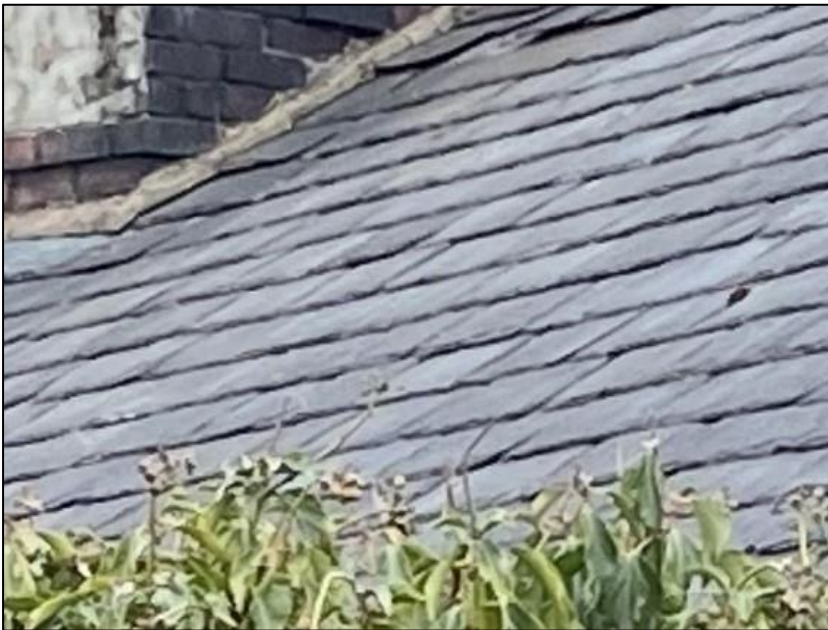
Photograph 10 showing the gaps under the slate tiles around the chimney
