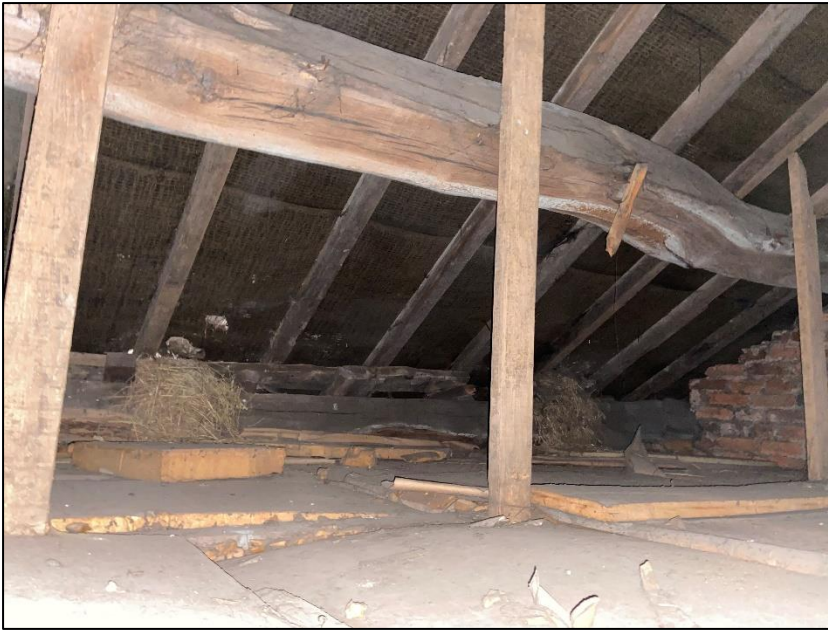
Photograph 14 showing the historic nesting material within the roof void.
