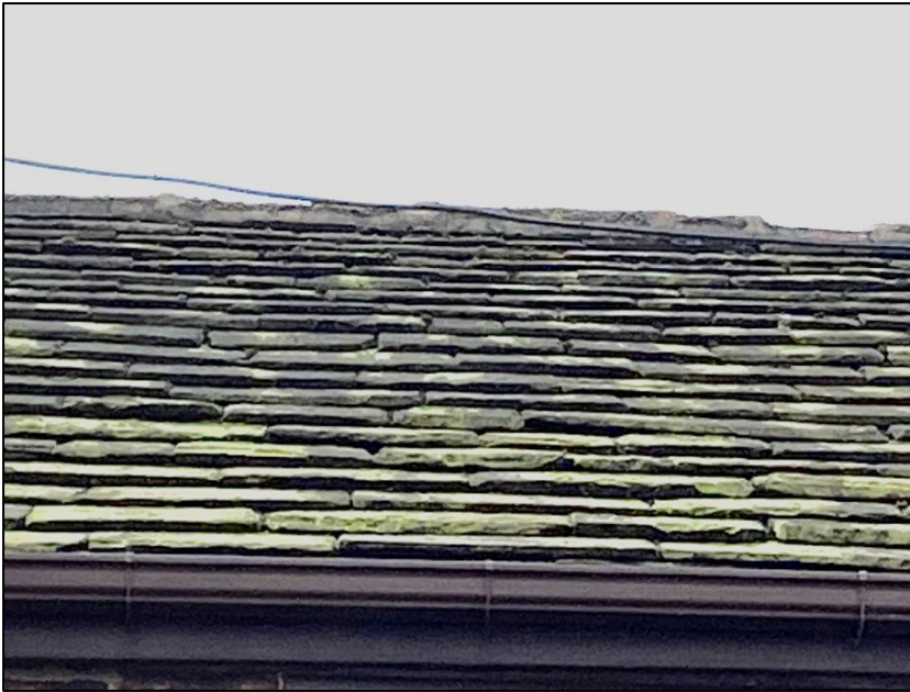
Photograph 9 showing the gaps under the stone tiles
