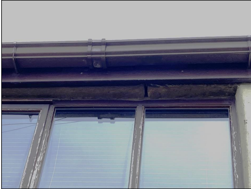
Photograph 8 showing the gap between two stones on the lintel
