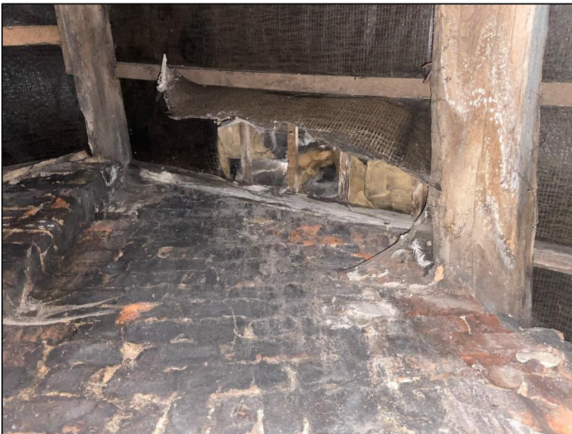
Photograph 12 showing the roof tiles behind an area of damaged roof lining material
