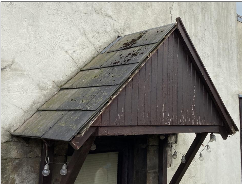
Photograph 7 showing the gap on the door canopy
