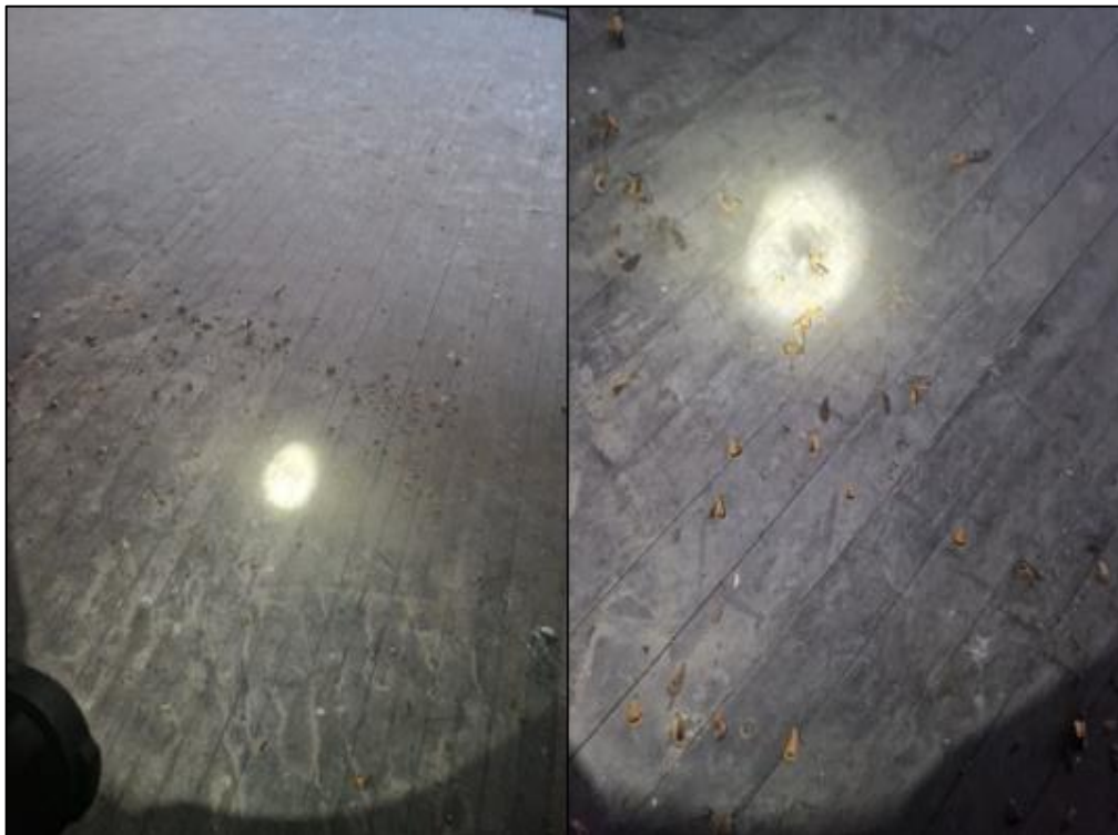
Figure 5.4 Pre-dusk inspection survey 1- Visual Aid – increased evidence of use by BLE, with feeding remains, dropping and splashing observed throughout the room.
