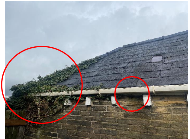
Photo 2: View of building one showing dense ivy at south western corner and gap under soffit.
