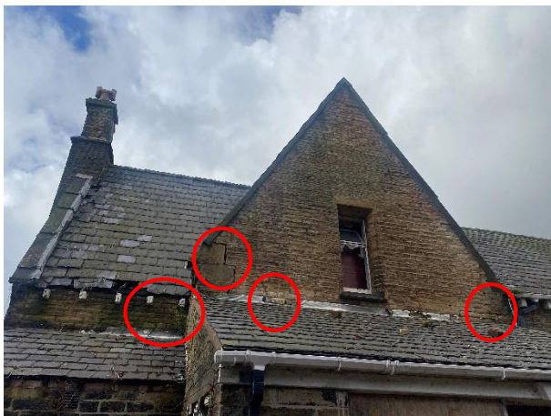
Photo 11: View of the eastern elevation of building two with missing mortar and damaged flashing.
