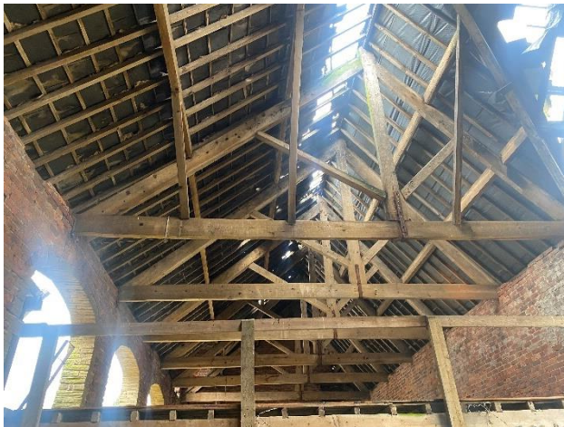
Photo 13: Internal view of major roof collapse on the western wing of building three.
