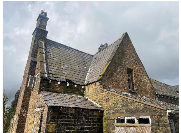
Photo 8: View from the south of building two showing numerous missing, lifted and slipped roof tiles.
