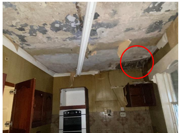
Photo 12: View of major hole in ceiling in building two leading to upper floor.
