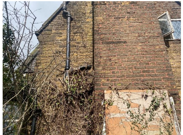
Photo 10: Area of dense ivy on the southern elevation of building two.
