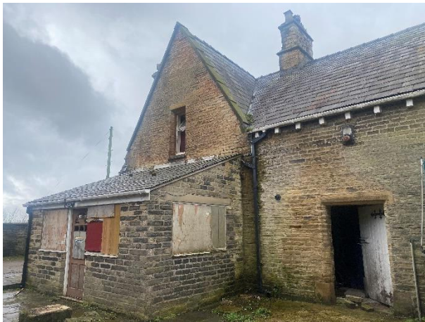
Photo 1: View of building two, showing general dilapidated nature of construction around the site.
