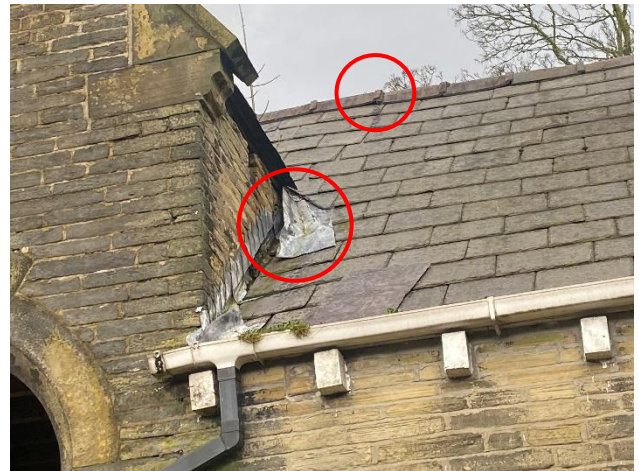
Photo 14: View of gap in ridge tile and lifted flashing on central dormer of the northern wing of building three.
