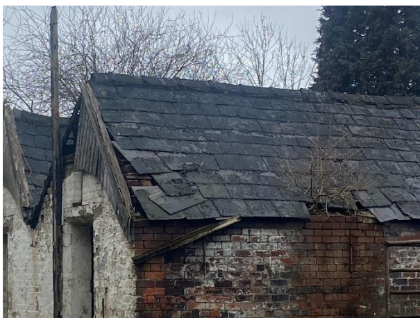
Photo 5: View of northern elevation of building one with innumerable areas of missing mortar and many slipped roof tiles.
