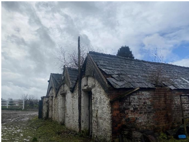
Photo 3: View of building one showing major gap in cladding, numerous areas of missing mortar, slipped roof tiles and extensive vegetation growth.
