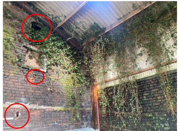
Photo 24: View of north eastern corner of building four showing dense ivy, missing bricks and major hole leading to building three.
