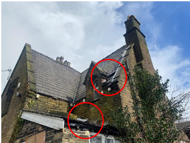
Photo 9: View from the west of building two showing areas of major roof collapse.
