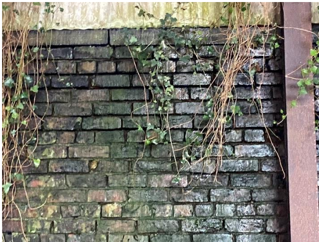
Photo 23: Close up of the eastern wall of building four showing extensive area of missing mortar.
