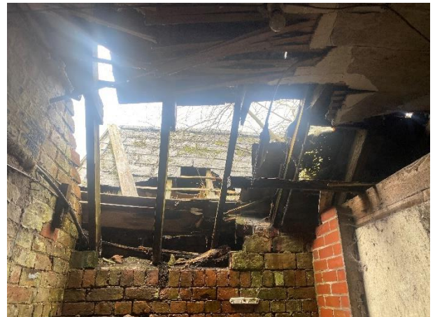
Photo 4: Major roof collapse on the central pitch of building one with numerous missing bricks and mortars.
