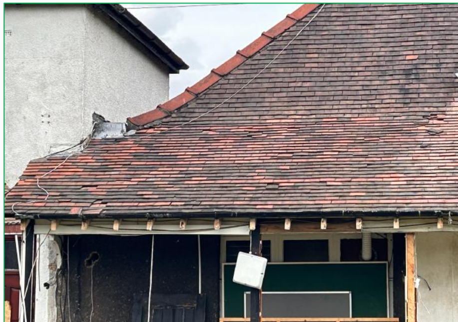
Showing slipped and missing tiles on the south elevation of the building
