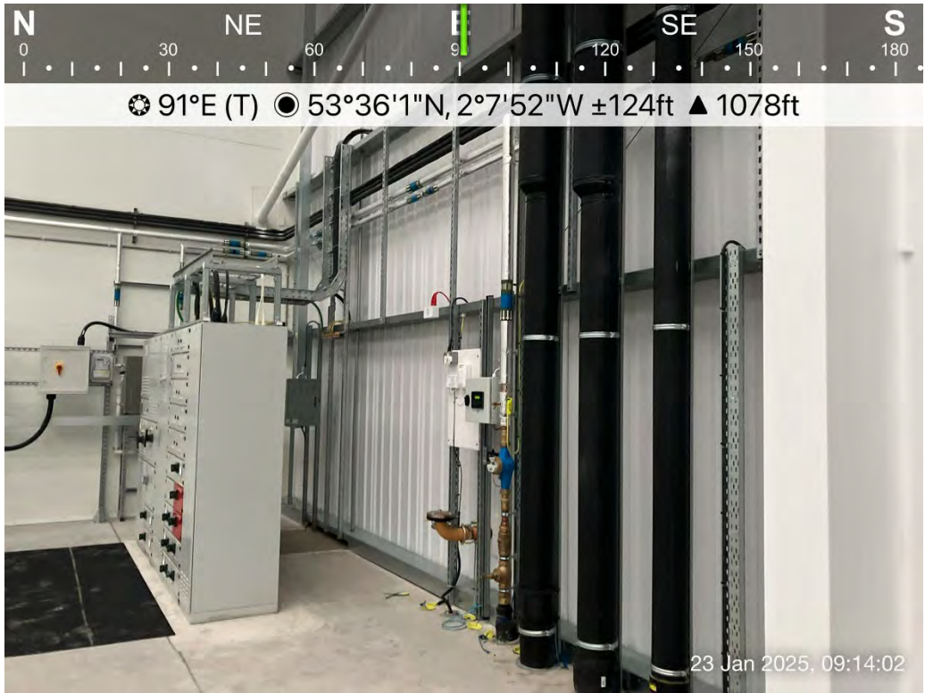
Photograph No.4: The electricity switchboard, gas input and potable water input are all located in the southeast of the building.
