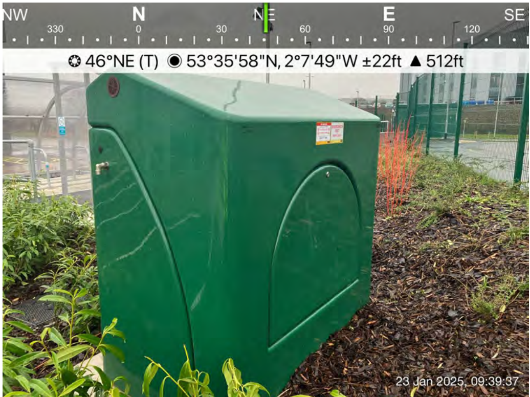
Photograph No.13: The gas meter is on the southern boundary of the site.
