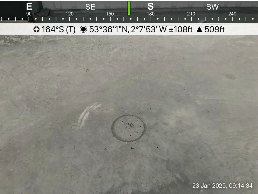
Photograph No.5: Markings and areas where the floor had been patched were noted across the warehouse floor.
