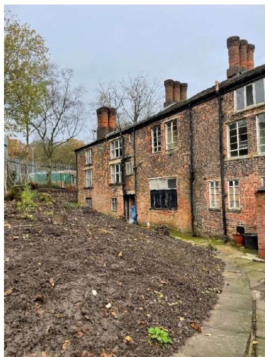
Figure 03 West wing of the building which is in a very unsafe condition
