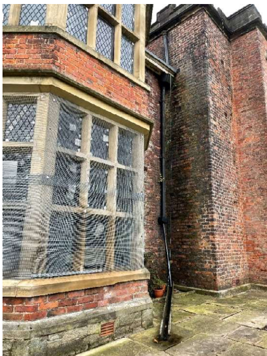
Figure 02 Rainwater pipe failure affecting the brickwork to the south-
