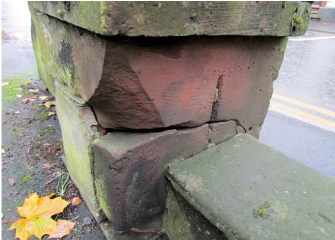
Damaged Corner of Base
