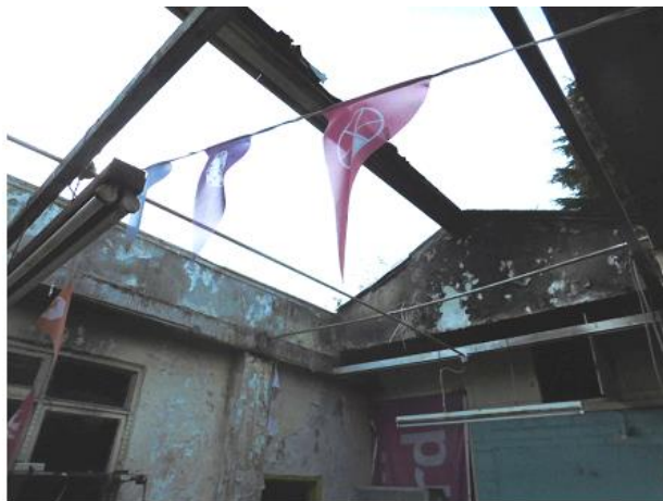
PHOTO 20 Missing Western Part of Building 2 Roof
