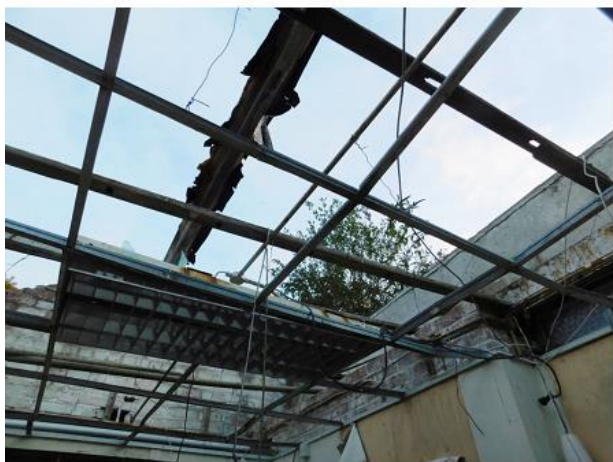
PHOTO 21 Missing Central Part of Building 2 Roof
