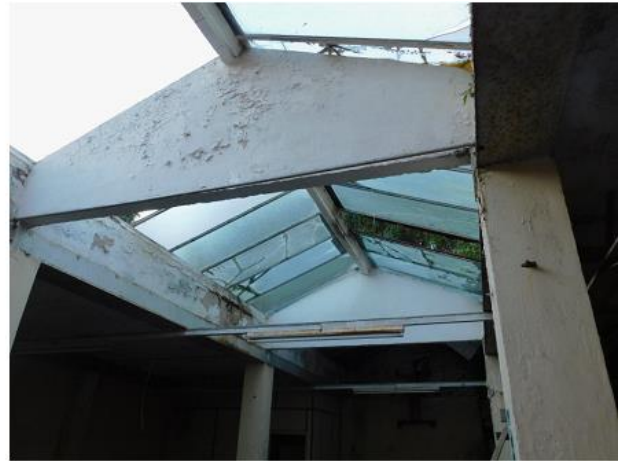
PHOTO 26 Missing Central Building 2 Roof
