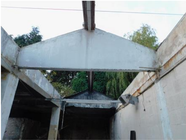
PHOTO 25 Missing Western Part of Building 2 Roof
