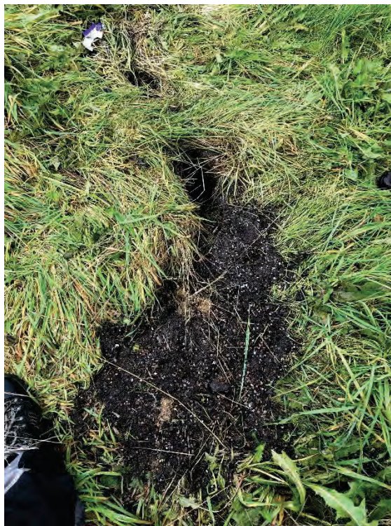
Photo 10: Evidence of infilled ground (2/2)
