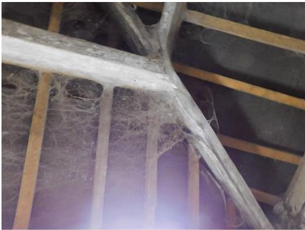
PHOTO 31 Underside of Cobwebs in Western Hip Roof
