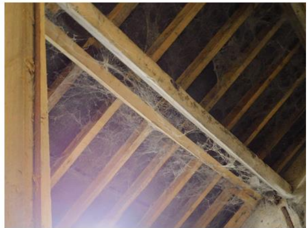
PHOTO 34 Cobwebs Along Internal Southern Roof Edge
