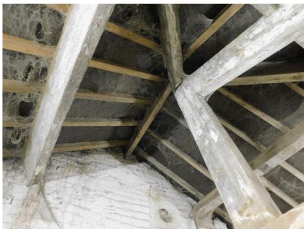
PHOTO 29 Cobwebs on Underside of Northern Roof
