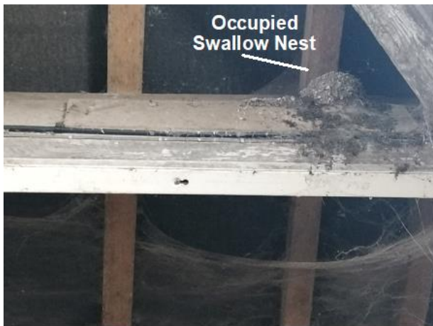
PHOTO 35 Nest in North-eastern Internal Roof Corner
