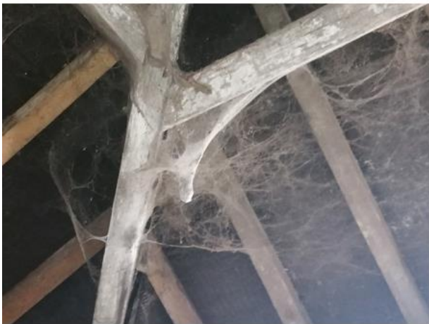
PHOTO 33 Collection of Cobwebs under Main Roof
