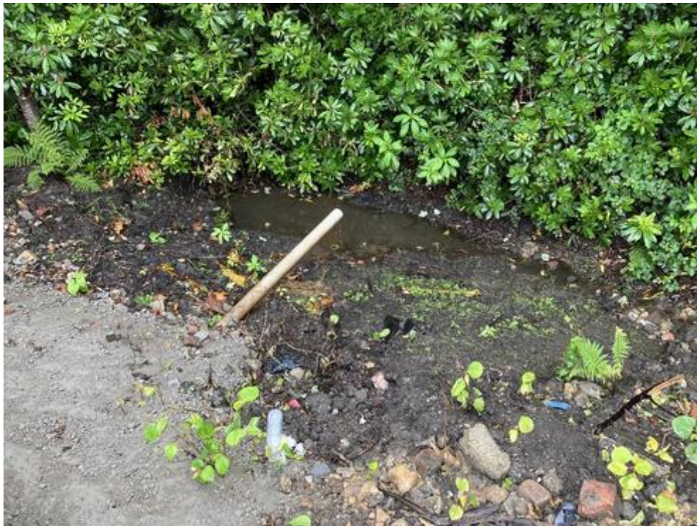
PLATE 8 DRAINAGE PIPE TO BROOK
