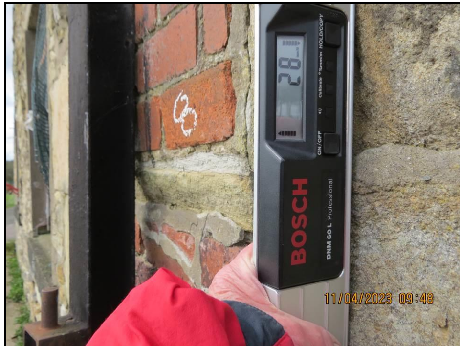
028 Loss of vertical alignment to gable, chainage 8.3 metres
