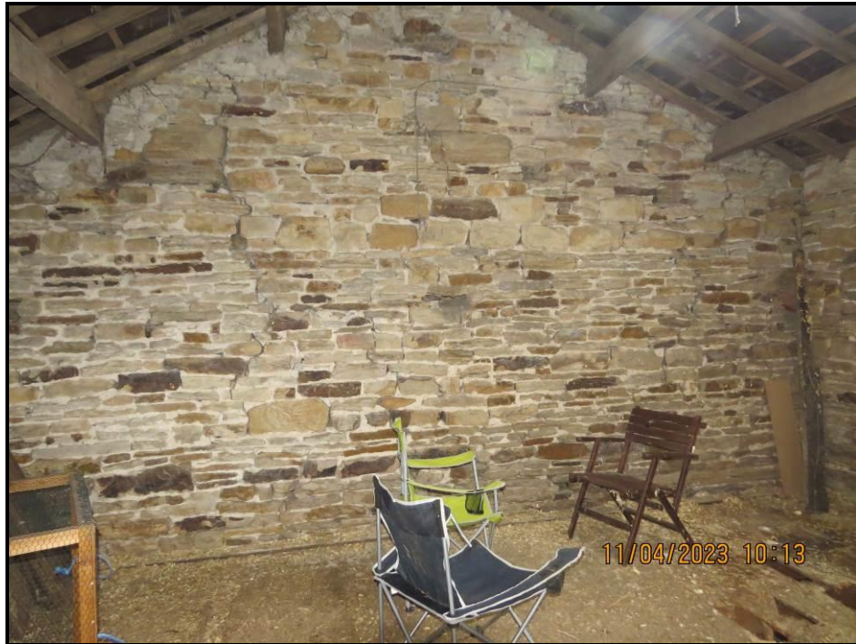
067 South East gable, historic crazing to gable
