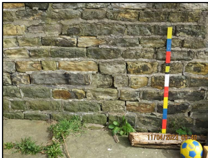
Photograph 015 Minor lateral movement (historic)
