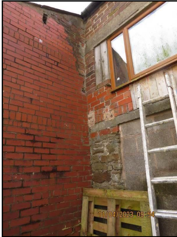
038 Satisfactory wall return
