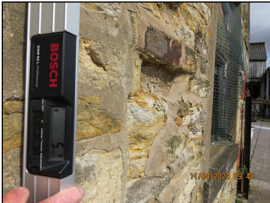
027 Loss of vertical alignment to gable, chainage 0
