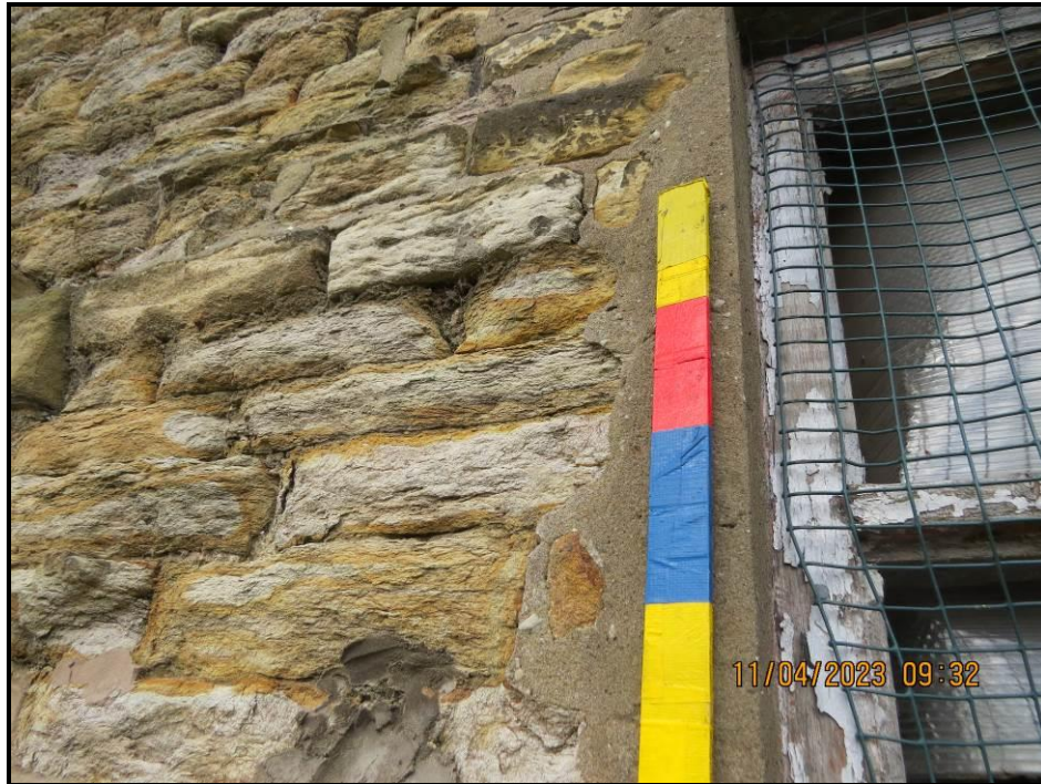
009 Weathering to stonework
