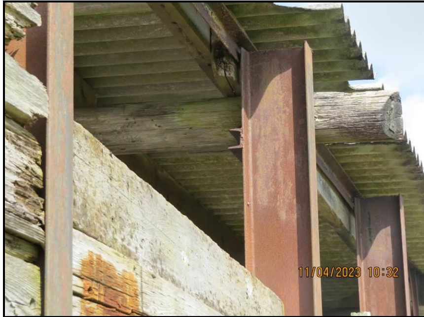
Photograph 087 Typical stanchion deformation
