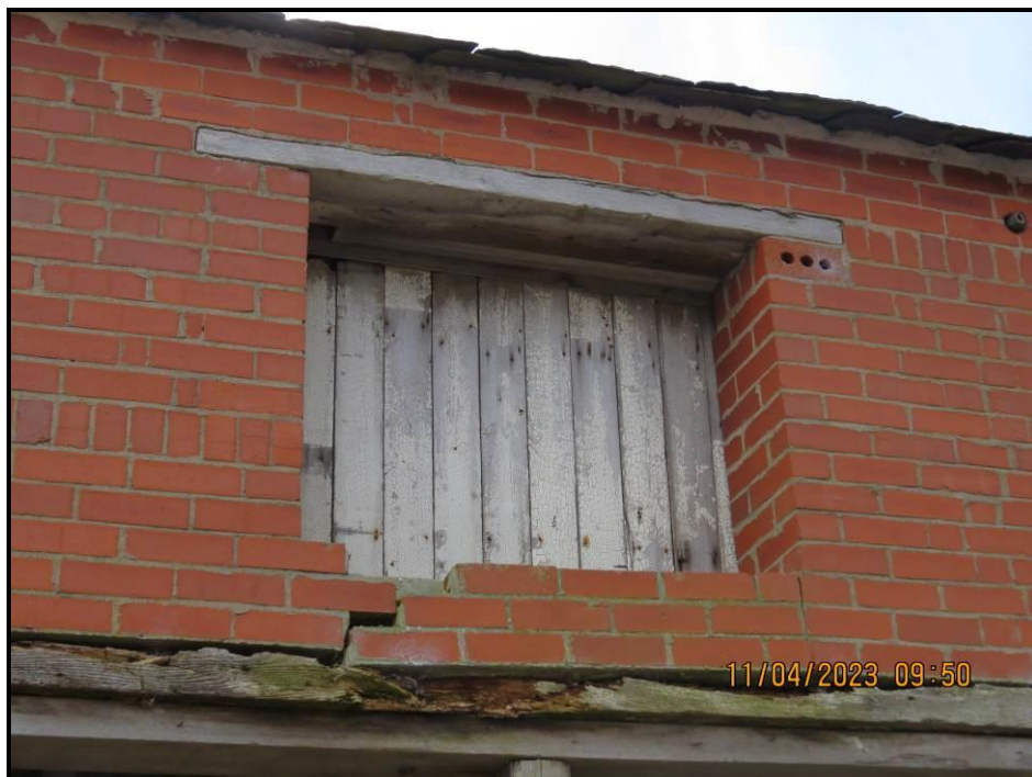
031 Lintel failure, cill collapse, chainage 0.5 – 3.3 metres
