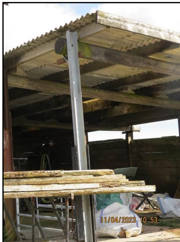
107 Irregular alignment to corner stanchion
