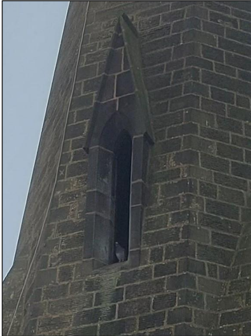
Fig.14- East facing window, with no louvres.
