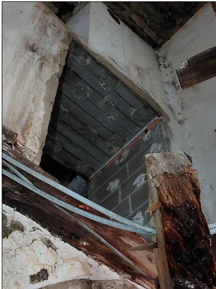
Fig.17 - View from ground floor within tower, through hole in first floor
