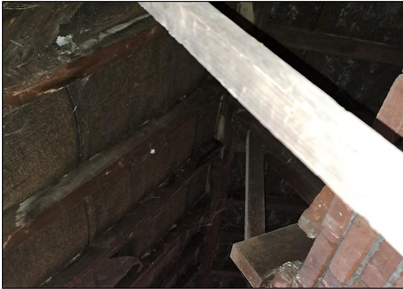
Photograph 9 showing a gap in the roof lining
