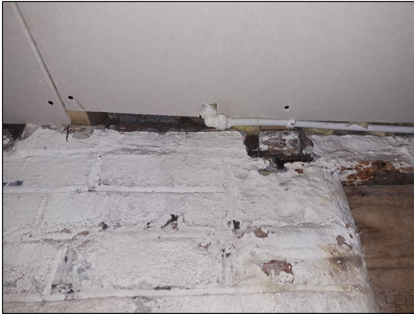
Photograph 13 showing a cavity in the stonework.
