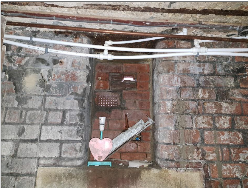
Photograph 12 showing a gap in the vent.
