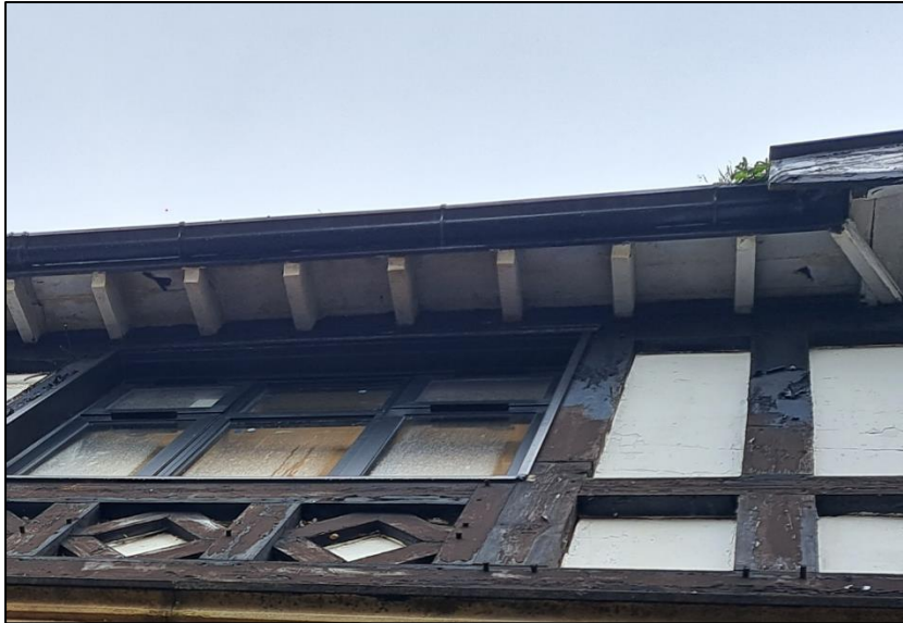
Photograph 3 showing gaps in the wooden soffit
