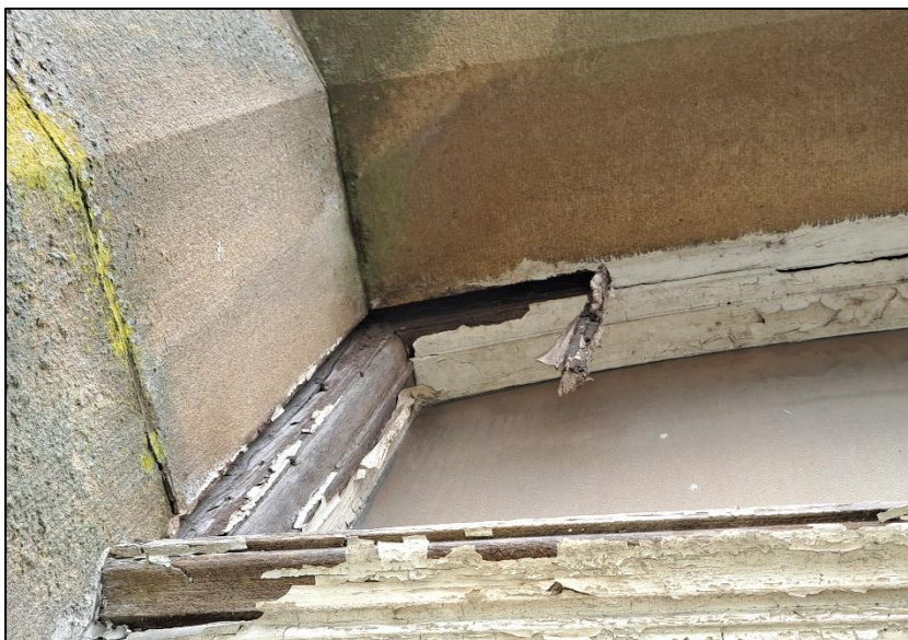
Photograph 6 showing a gap in the lintel.
