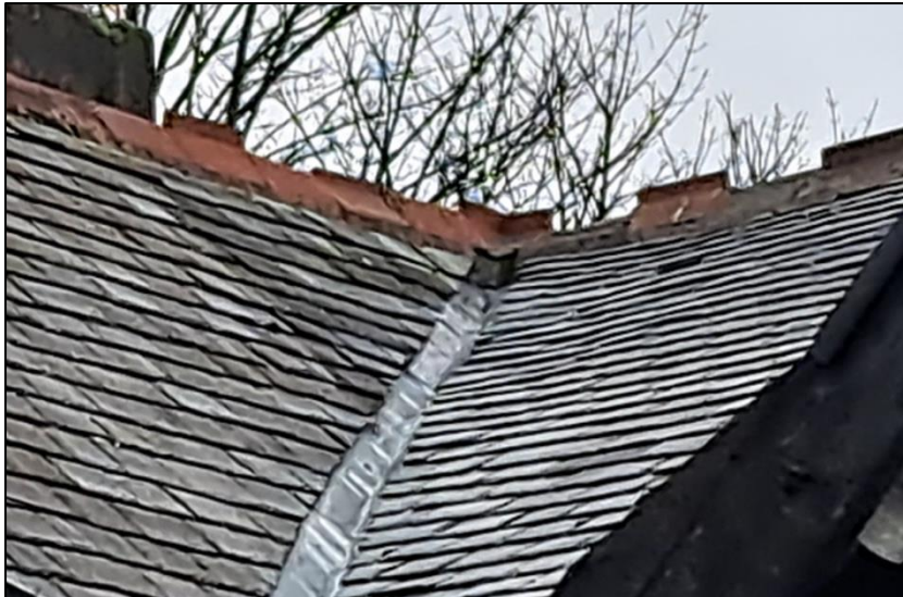
Photograph 5 showing slipped and damaged slate tiles.
