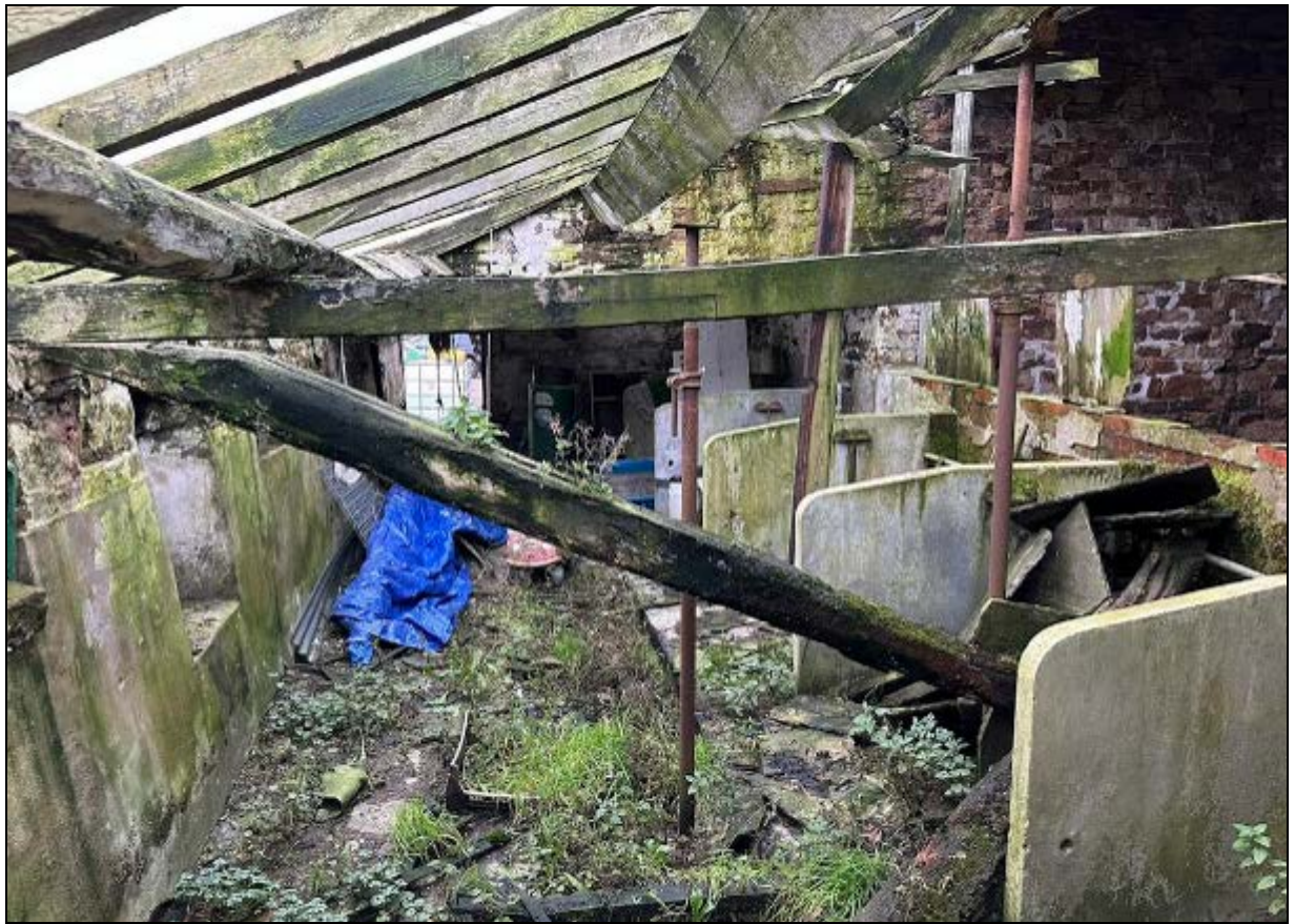
11, Derelect interior of the long outshut
