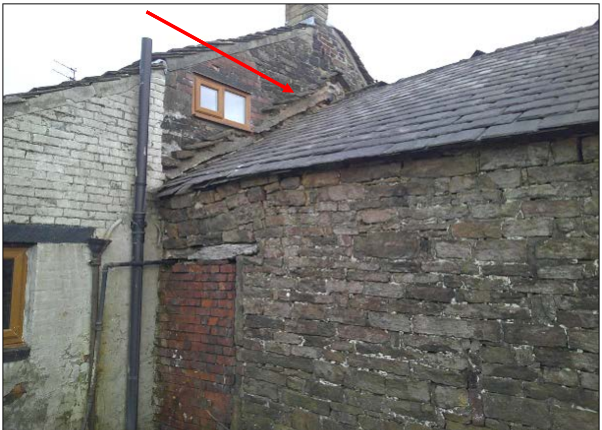
6. Blocked door in west elevation of the barn and redundant water tabling (indicated)
