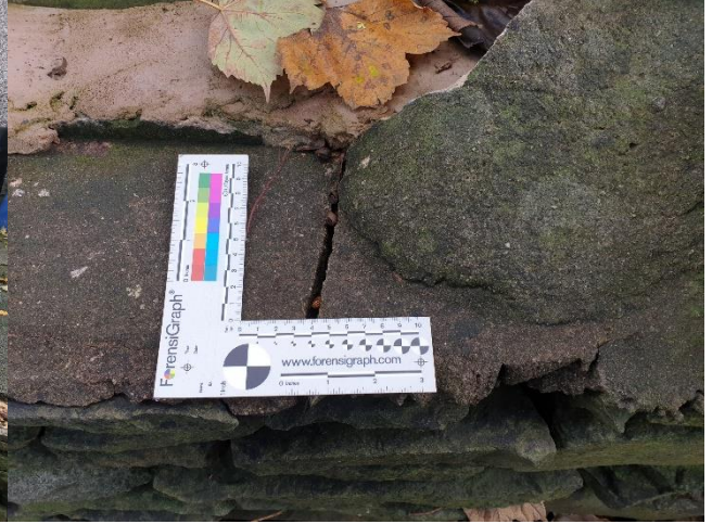
Photo 3: Crack in edge of steps
