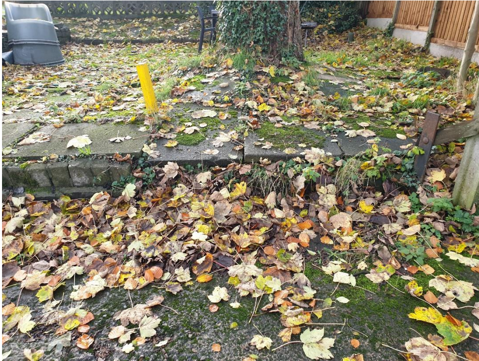
Photo 1 – Lifting of slabs adjacent to trunk, cracked mortar, uneven surfaces
