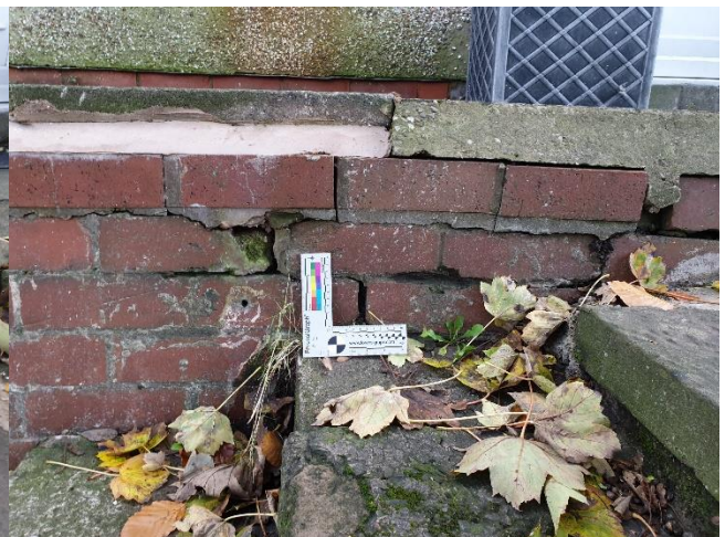
Photo 5: Existing cracks in brickwork
