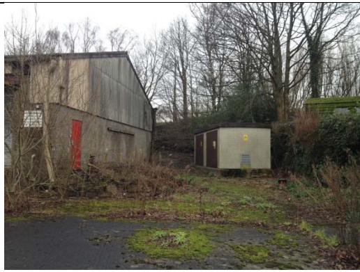
Photograph 2 (P2) Electrical substation to the east of the former Works building.
