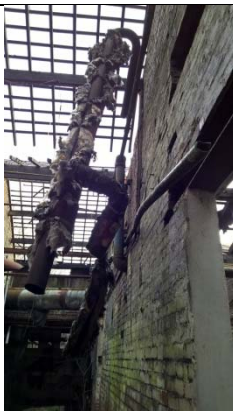
Photograph 10 (P10) Suspected ACM such as pipe lagging were noted to be in poor condition.
