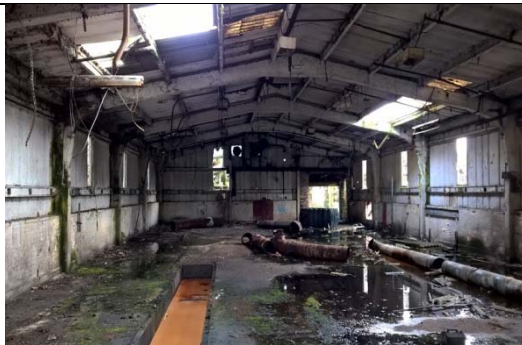
Photograph 7 (P7) Former hydraulic press area with visible evidence of contamination.
