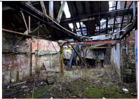
Photograph 9 (P9) Former Works building is significantly damaged and mostly inaccessible.
