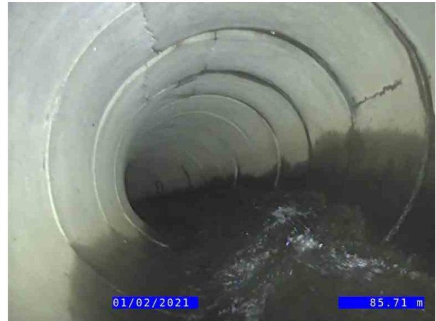
INLET 1X_81bb722b-2072-4e85-8e8e-064e5d7a3a6f_20210203_13 0607_530.jpg, 00:04:18, 85.71 m Crack, longitudinal at 12 o'clock, start
