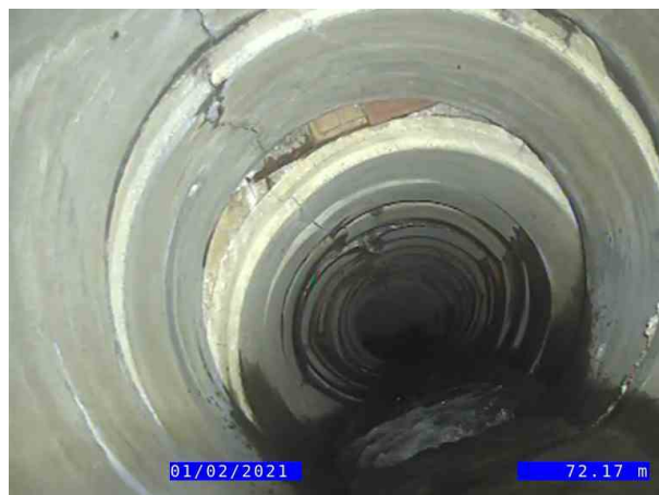
INLET 1X_c6e62192-60a6-490d-81de-857f7a6a7a6b_20210203_130 444_484.jpg, 00:03:43, 72.17 m Open joint, large
