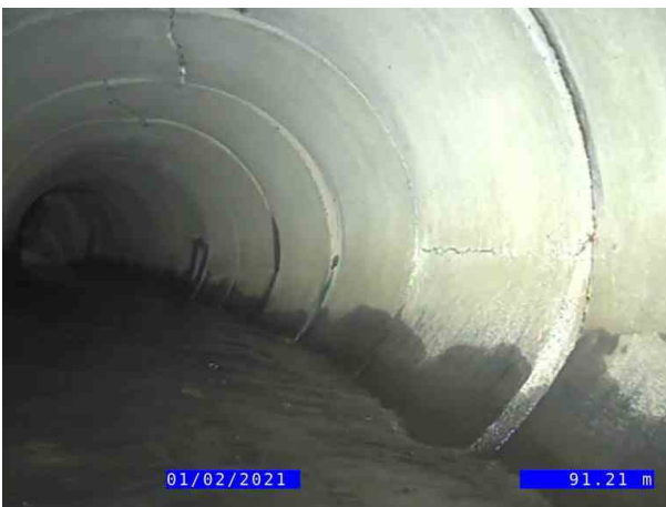
INLET 1X_e6707430-7b58-4a34-af85-04722aaecef2_20210203_130 628_953.jpg, 00:04:30, 91.21 m Crack, longitudinal at 3 o'clock
