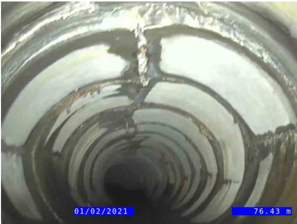
INLET 1X_0eb6446b-83ab-439b-a7f2-4e50c1710dc5_20210203_130 543_451.jpg, 00:03:58, 76.63 m Infiltration, dripping at 12 o'clock
