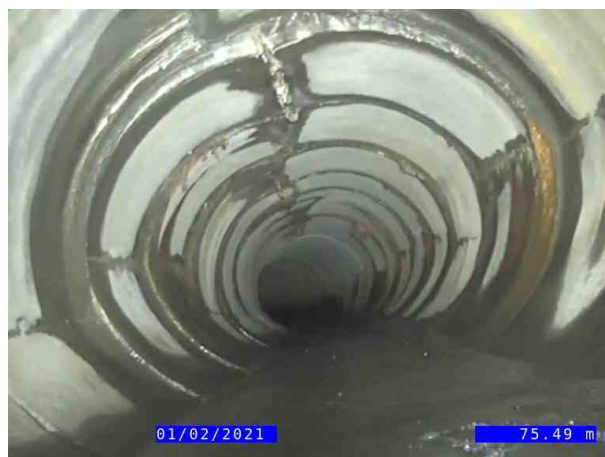
INLET 1X_fe46afd1-a152-4f45-ab7a-3a2f78f05362_20210203_1305 22_603.jpg, 00:03:55, 75.49 m Fracture, multiple from 8 o'clock to 4 o'clock, start
