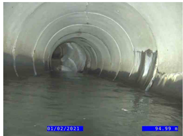
INLET 1X_fc4a4ff4-8edf-45ab-ad75-d9d1db5816f7_20210203_1306 44_636.jpg, 00:04:39, 94.99 m Crack, longitudinal at 3 o'clock
