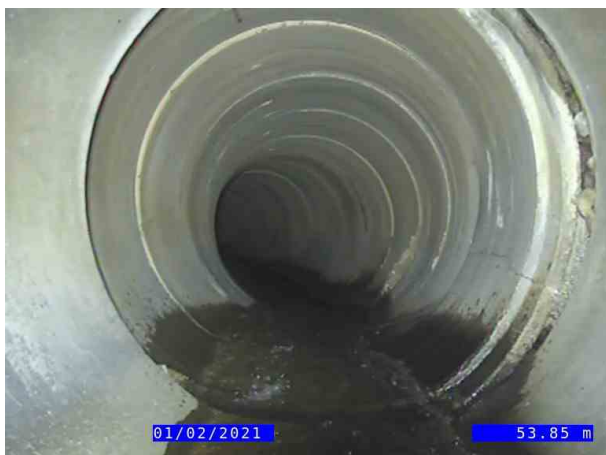
INLET 1X_7c5fd752-22c8-4d4c-ac4a-4a40e8247a25_20210203_124 047_518.jpg, 00:02:55, 53.85 m Open joint, medium
