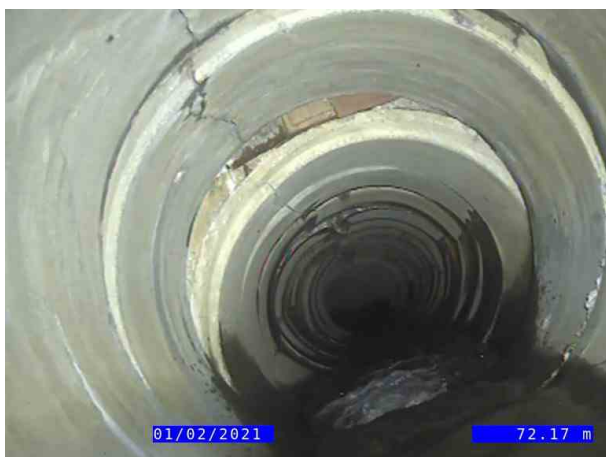
INLET 1X_312eb7a8-8247-4b52-af81-2483cd2e0f71_20210203_130 453_700.jpg, 00:03:43, 72.17 m Crack, longitudinal at 12 o'clock
