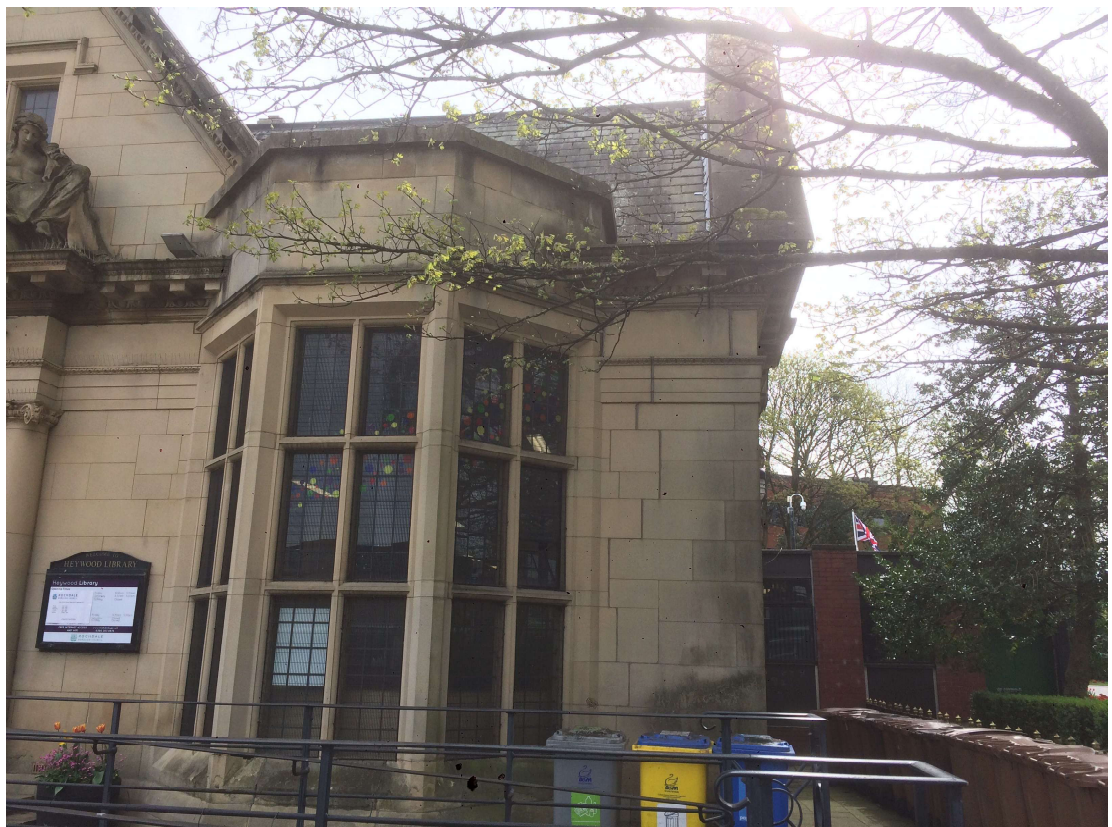
Front Elevation Right Side, Open Joints
