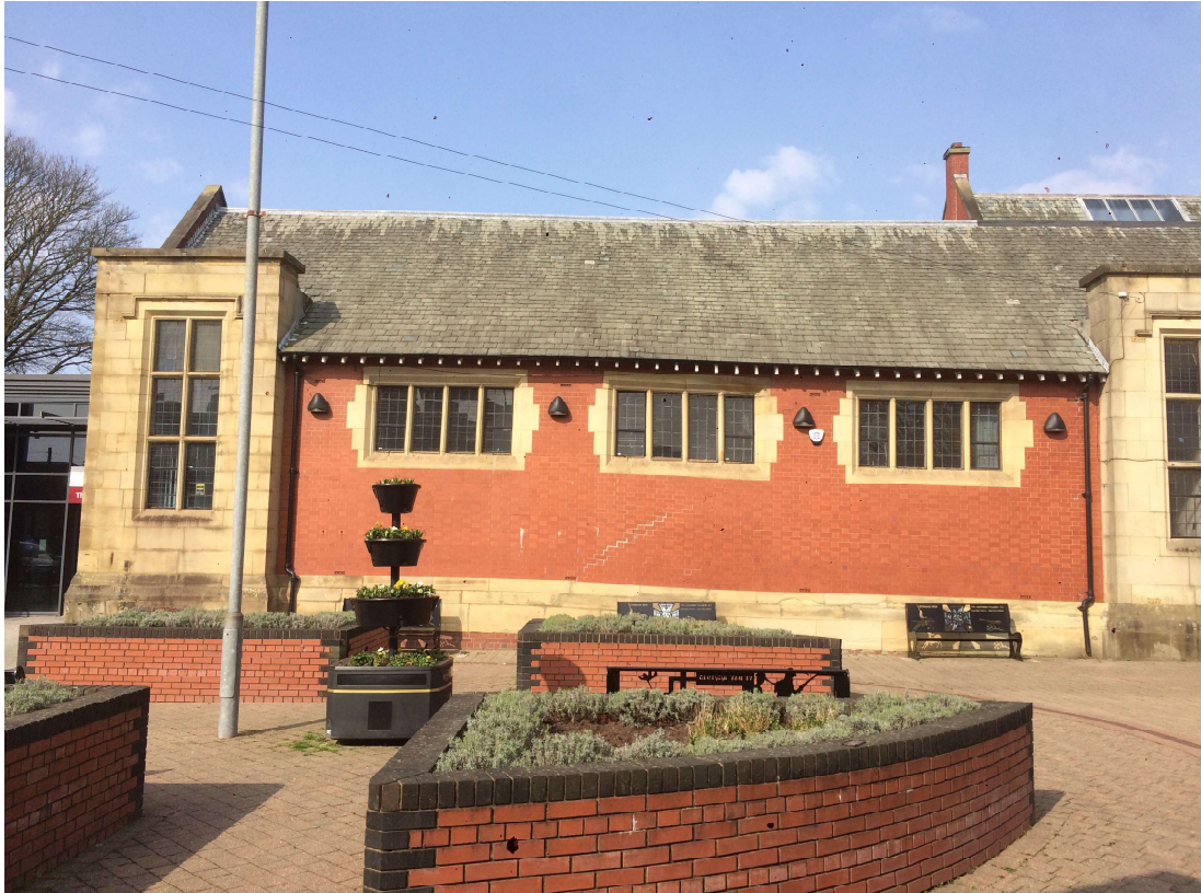
West Elevation Showing Settlement
