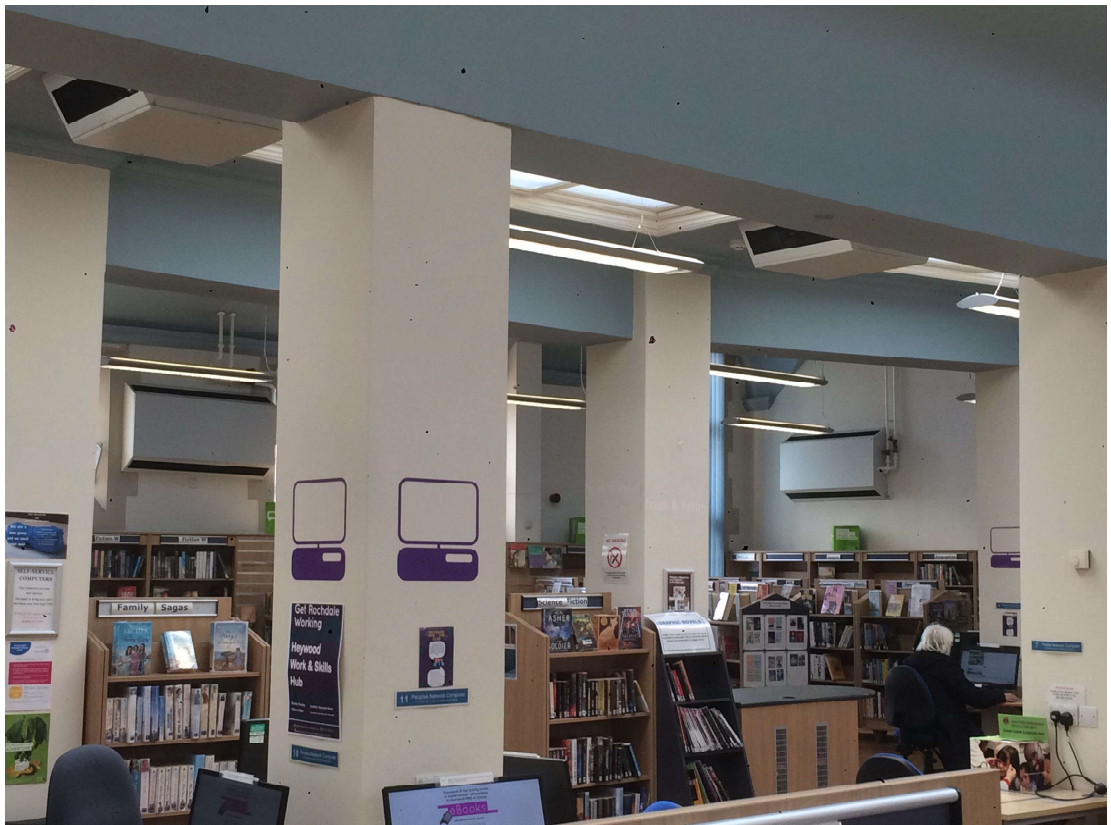
Interior, Showing Settlement of Columns
