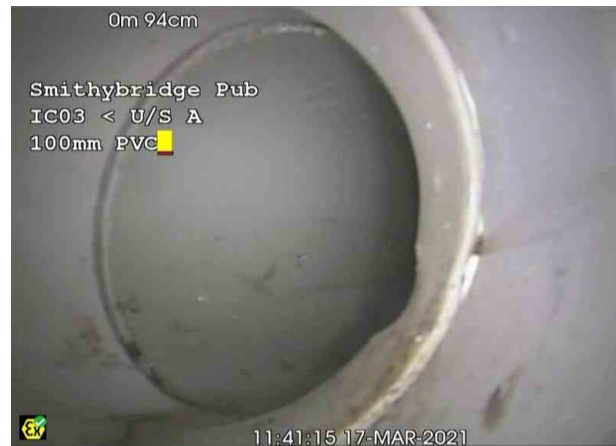
IC03 U_S AX_9e3a0a8c-97fe-463f-90c9-c8c96d97aafc_20210326_1150 41_713.jpg, 00:00:07, 0.94 m Line deviates right, Approx 90 degrees
