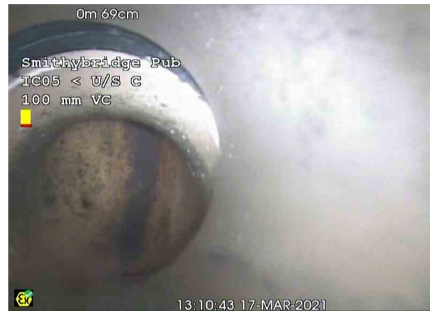
IC05 U_S CX_3d9348c4-45f9-4fe4-848a-202ea901d854_20210326_123 358_614.jpg, 00:00:05, 0.69 m Joint displaced, large, Band seal visible
