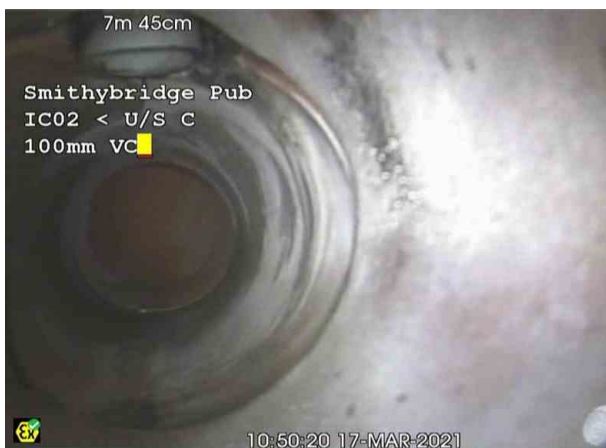
IC02 U_S CX_70b95ca6-0eb4-4064-962c-fb0f0544179a_20210326_095 853_176.jpg, 00:00:42, 7.45 m Connection other than junction at 12 o'clock, diameter: 25mm
