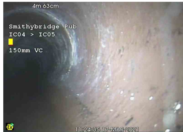
IC04X_8cc0c8f9-5257-4923-83f0-b68e224434c7_20210326_1 13209_390.jpg, 00:00:42, 4.63 m Junction at 10 o'clock, diameter: 100mm
