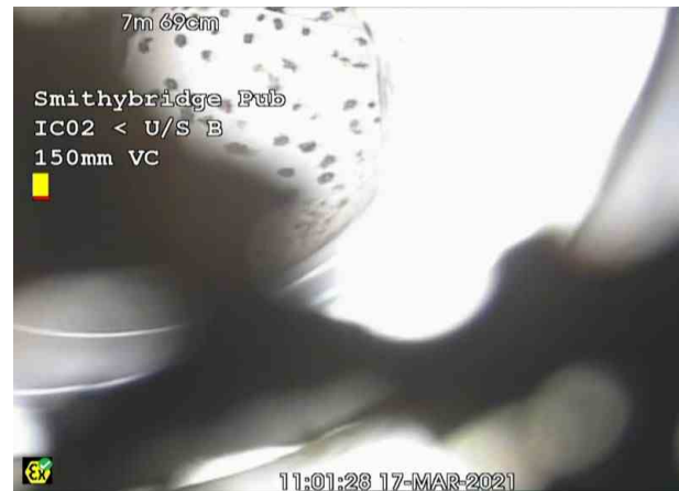
IC02 U_S BX_d2a3e845-ad65-413e-8335-d81d7f5fc821_20210326_111 111_904.jpg, 00:01:13, 7.69 m Finish node, other special chamber, reference: IC02 U/S B, Waste discharge point
