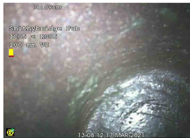
RG05X_d87ac500-43ab-4f26-b197-79fe25f380a9_20210326_121708_757.jpg, 00:01:03, 7.89 m Finish node, gully, reference: RG05
