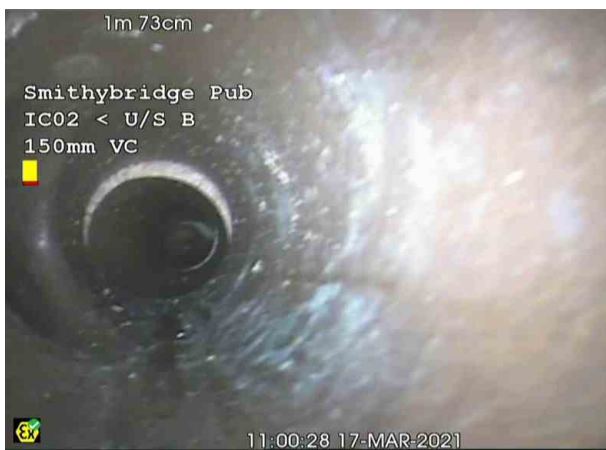
IC02 U_S BX_ff442f2-28d4-438b-82ea-4f5a3b9cefeb_20210326_11081 1_071.jpg, 00:00:13, 1.73 m Junction at 8 o'clock, diameter: 100mm
