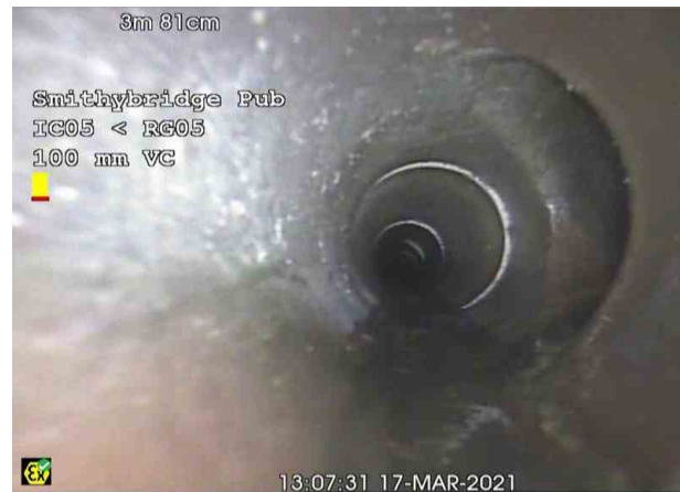
RG05X_1d0c6782-b4f7-462f-9fe1-2de1d3ea2e99_20210326_121330_977.jpg, 00:00:21, 3.81 m Junction at 3 o'clock, diameter: 100mm
