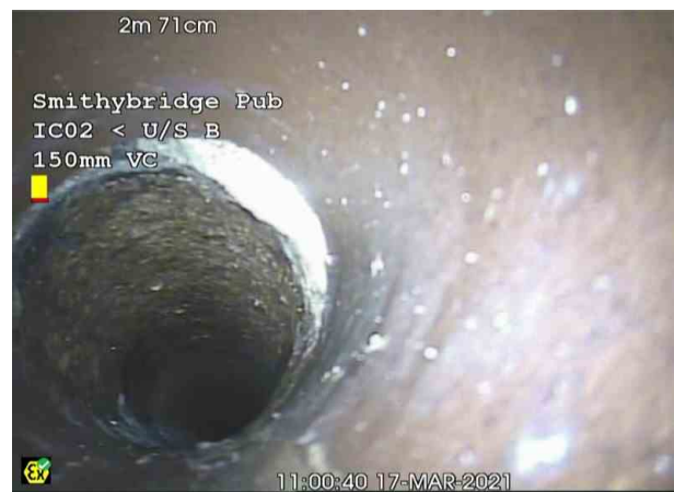
IC02 U_S BX_242ec4b5-9145-4bb9-b8d8-355af8a53835_20210326_110 943_193.jpg, 00:00:24, 2.71 m Pipe material changes to cast iron at this point
