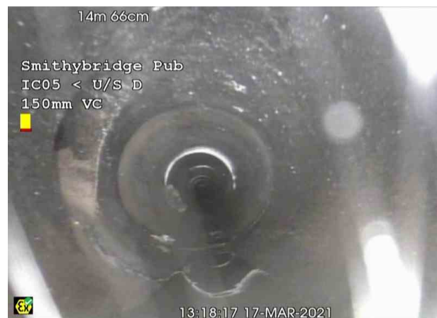
IC05 U_S DX_e578da2d-5c77-4bc2-861b-8a0ae9aaa63c_20210326_123 935_093.jpg, 00:01:27, 14.66 m Junction at 10 o'clock, diameter: 100mm
