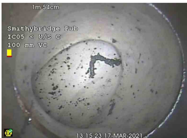
IC05 U_S CX_ffba0a50-97c4-4a54-96ec-78fb6d810f9b_20210326_1235 33_219.jpg, 00:01:59, 1.54 m Finish node, other special chamber, reference: IC05 U/S C, Waste discharge point
