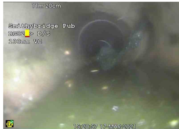
RG02X_d90418a4-f563-4736-bd08-961766937f07_20210326_135910_556.jpg, 00:05:33, 11.20 m Roots, tap, from junction
