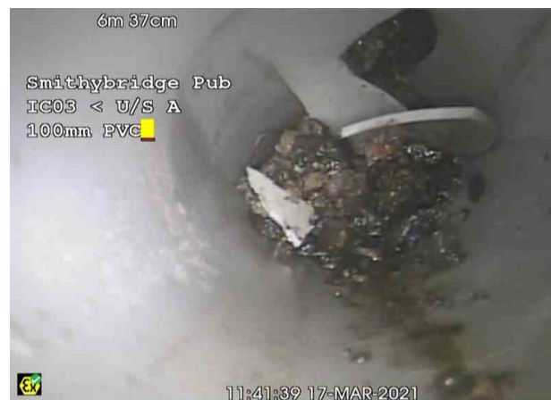
IC03 U_S AX_eedd93d8-598c-4417-91fb-52df387d14ff_20210326_1153 22_382.jpg, 00:00:31, 6.37 m Hole in drain or sewer from 12 o'clock to 3 o'clock
