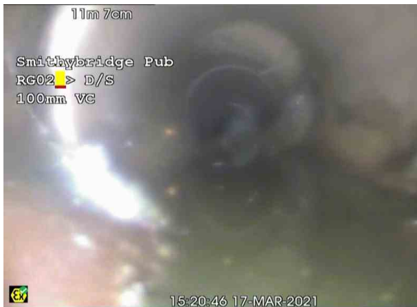
RG02X_63dd7449-0cd9-4f5b-8a10-e60ffb3a7324_20210326_135601_131.jpg, 00:05:22, 11.07 m Junction at 2 o'clock, diameter: 100mm
