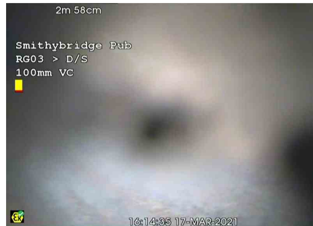
RG03X_11130214-9649-436d-94f8-bf45aaf29857_20210326_141811_497.jpg, 00:00:47, 2.58 m Finish node, other special chamber, reference: RG03 D/S, T Junction
