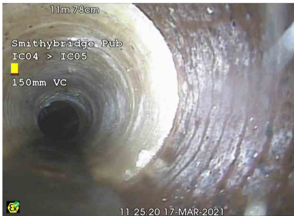
IC04X_bb2fe570-7059-4250-9fdb-52abdbfb31b6_20210326_1 13346_864.jpg, 00:01:26, 11.78 m Surface damage, corrosion products from 12 o'clock to 12 o'clock, start
