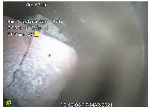
IC02 U_S DX_981bfd3d-3bfb-4873-b6a9-a4d86b7b5449_20210326_105 043_537.jpg, 00:00:10, 0.67 m Survey abandoned, Capped off Not in use
