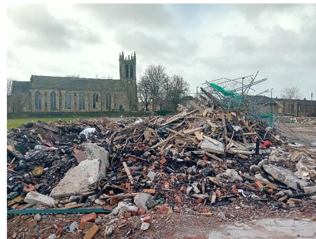
Photo 4: Rubble pile at target note TN1.
