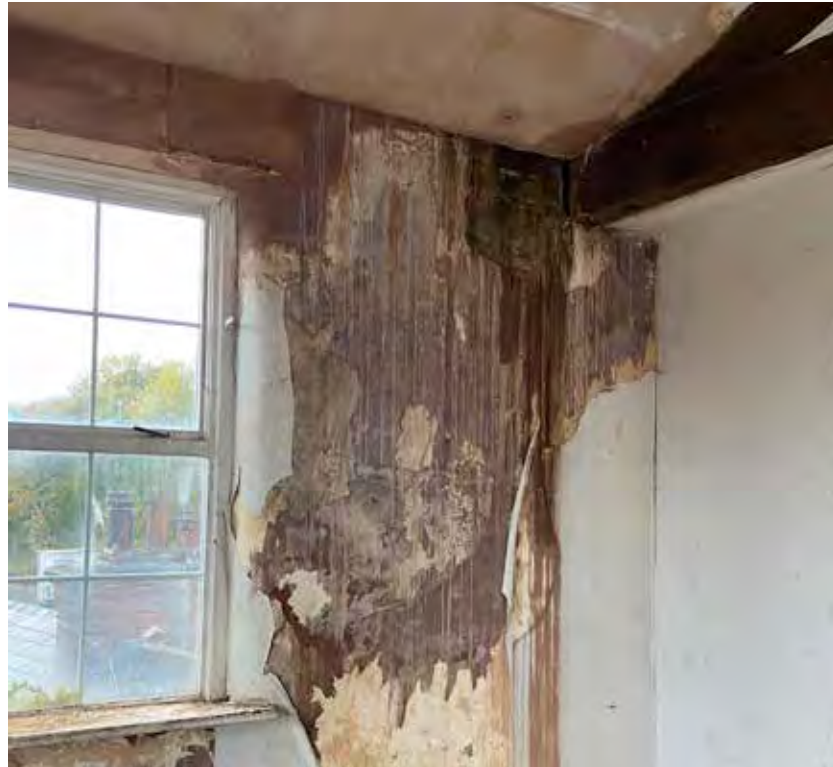
4.13a Damp in Ceiling due to roof failure
