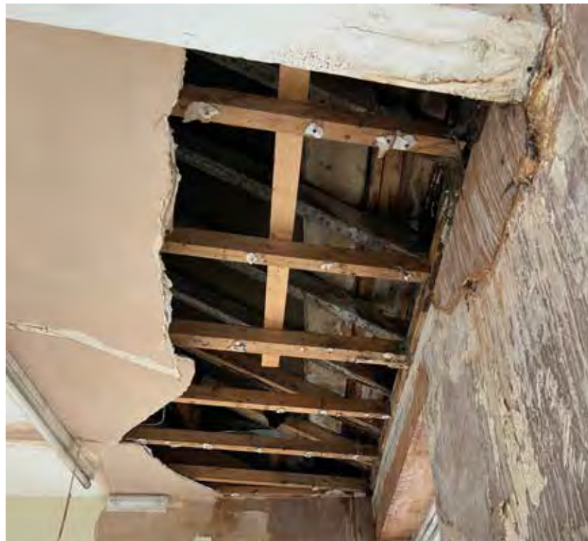
4.14 Water ingress to ceiling and rotting timbers
