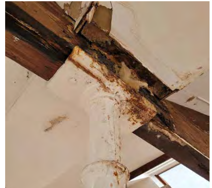
4.16 Water ingress damage to cast iron columns
