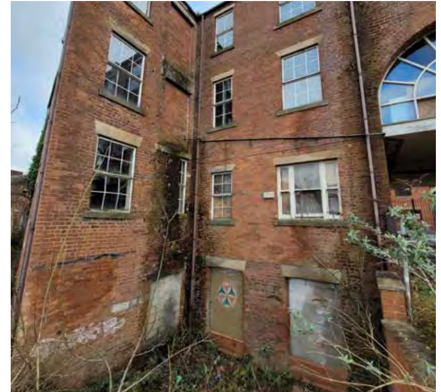
4.13c Water damage due to failing rainwater goods
