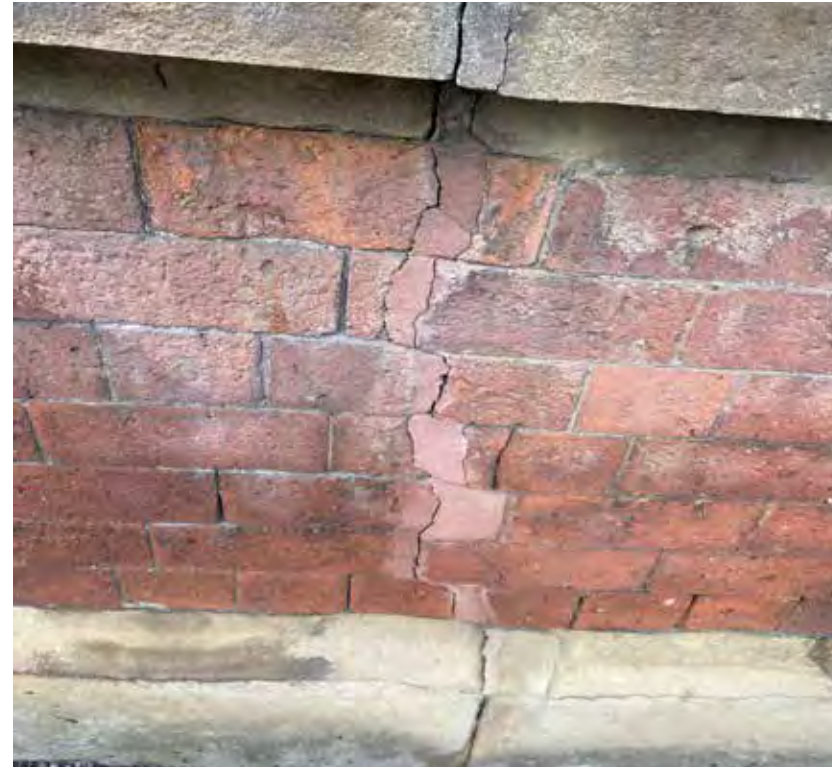
4.13b Cracking to South Elevation & friable masonry
