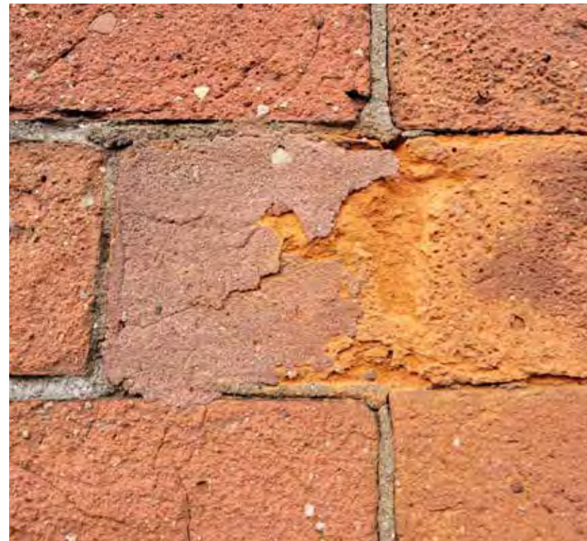
4.15 Damaging cementitious repairs to South Elevation
