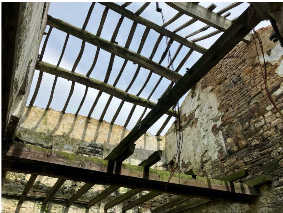
Photo 17: Bay 6 - Roof & First Floor Structure in Poor Condition
