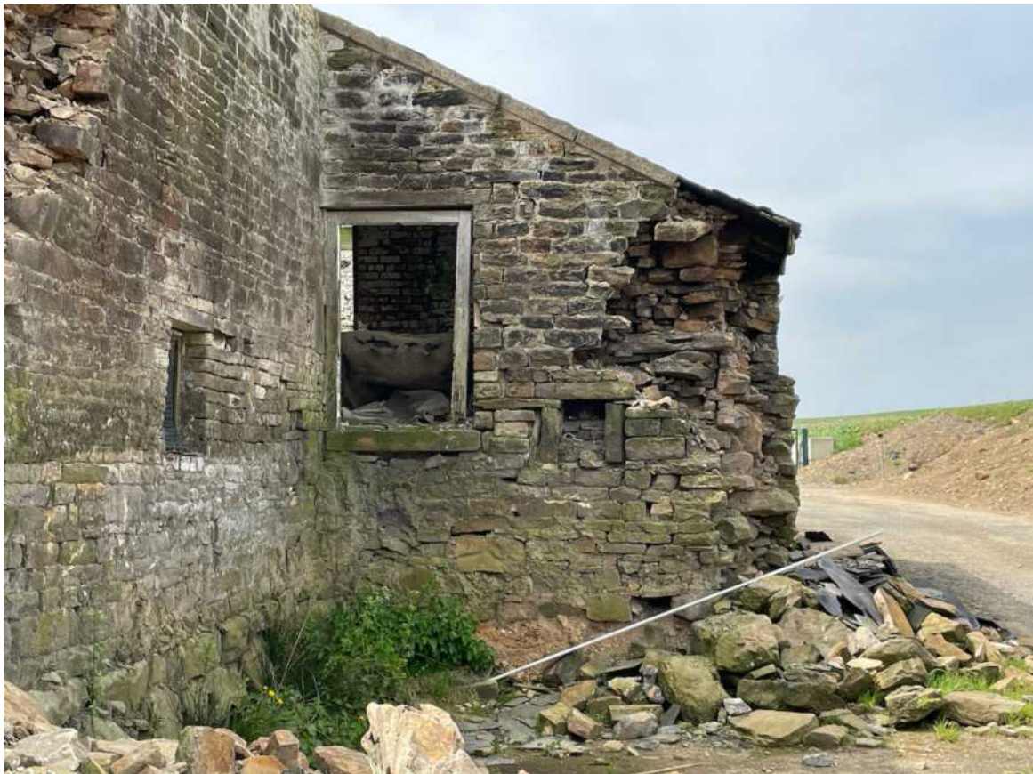
Photo 5: Lean-To Extension – Collapsed Masonry
