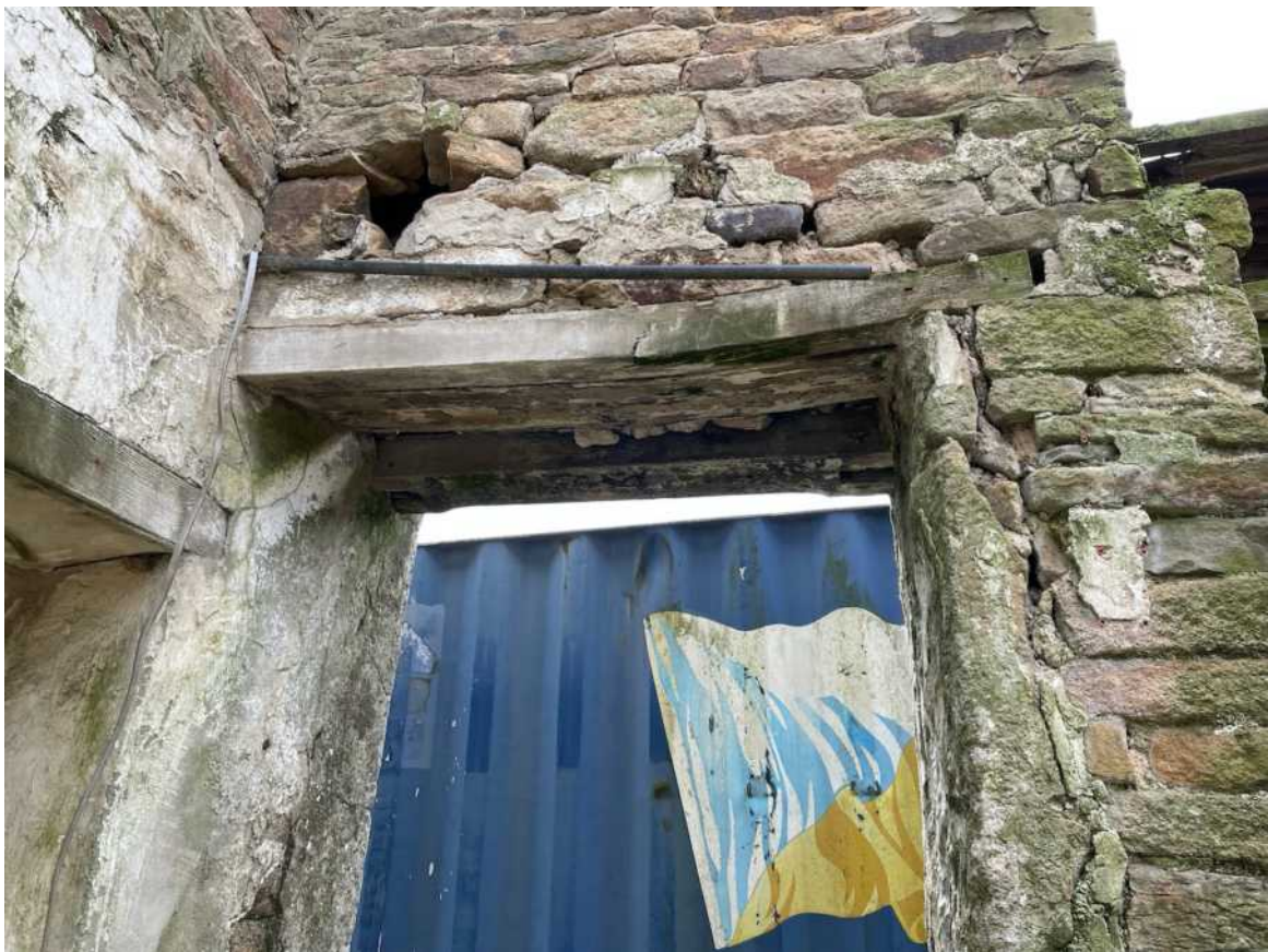
Photo 11: Failing Timber Lintels
