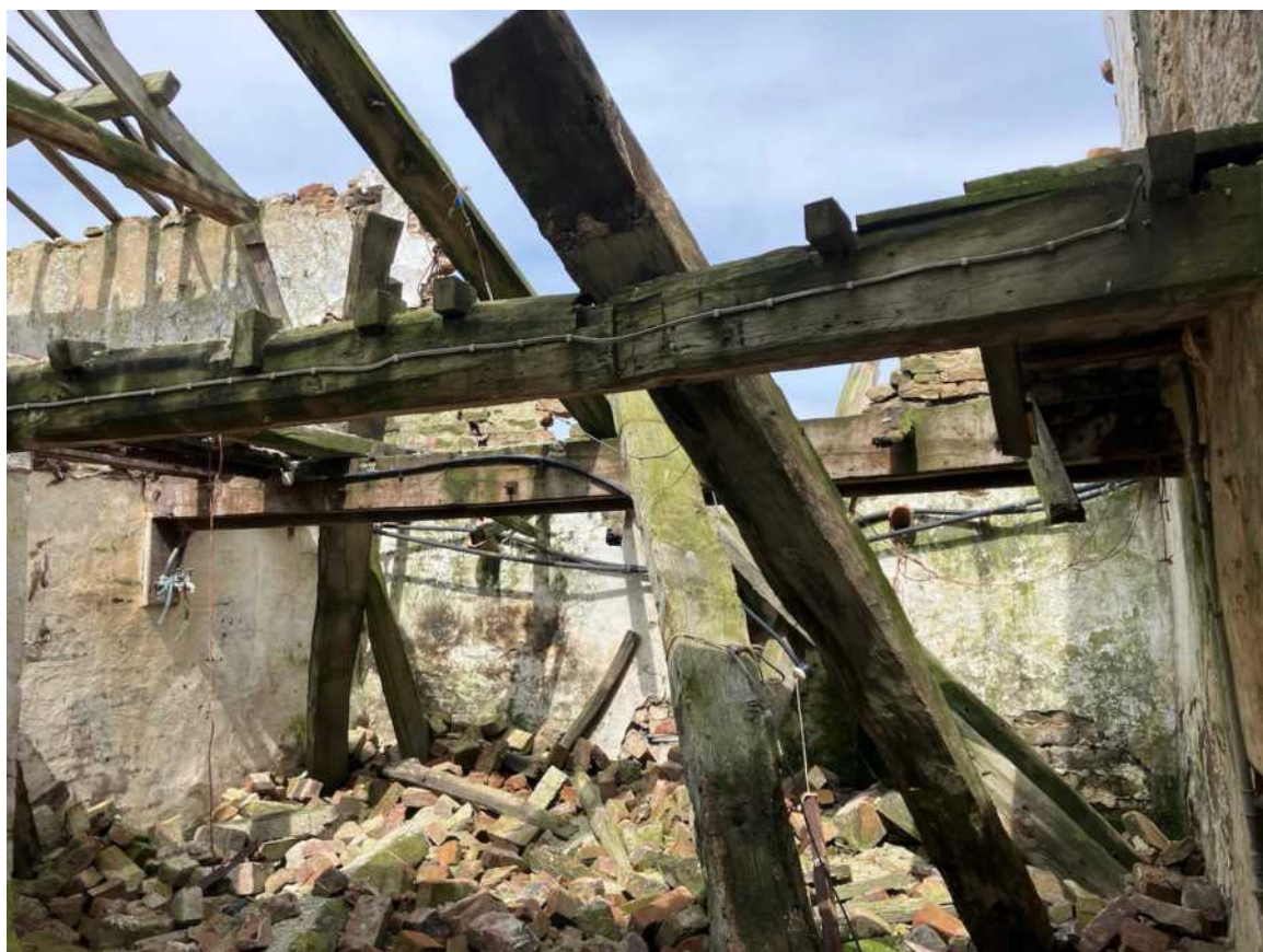
Photo 16: Bay 5 - Collapsed Roof & First Floor Structure
