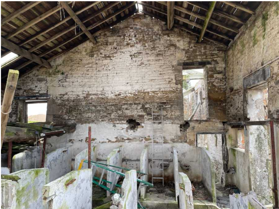
Photo 14: Bay 3 - Roof Structure & Missing First Floor
