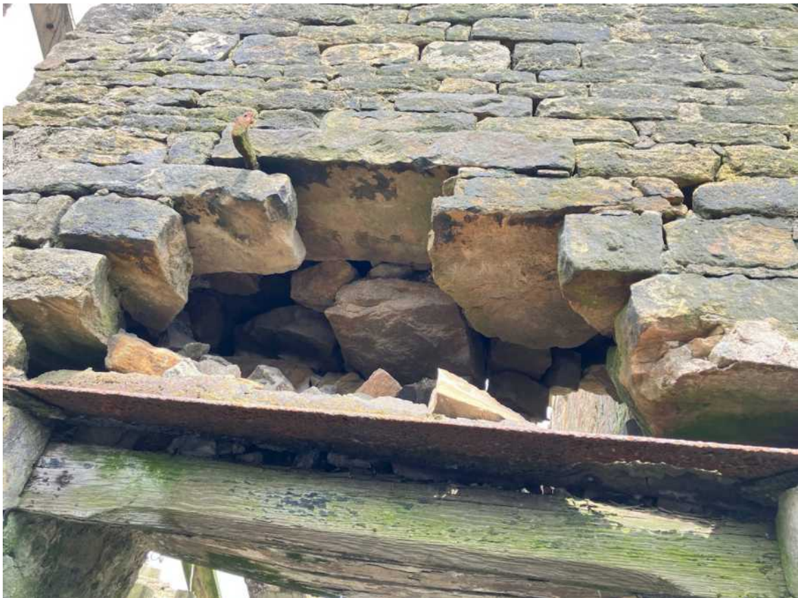
Photo 12: Missing Outer Facing Over Failing Timber Lintels
