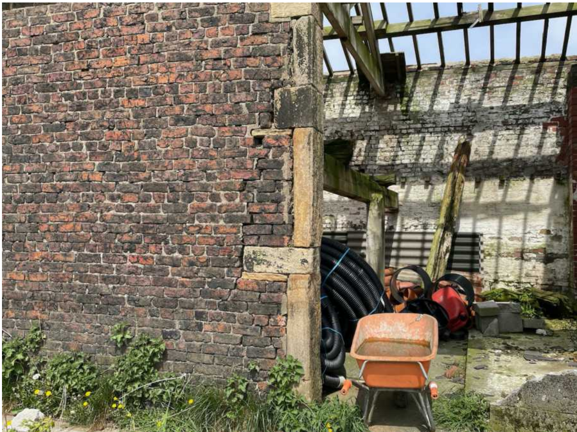
Photo 10: Cart Entrance - Vertical Cracking
