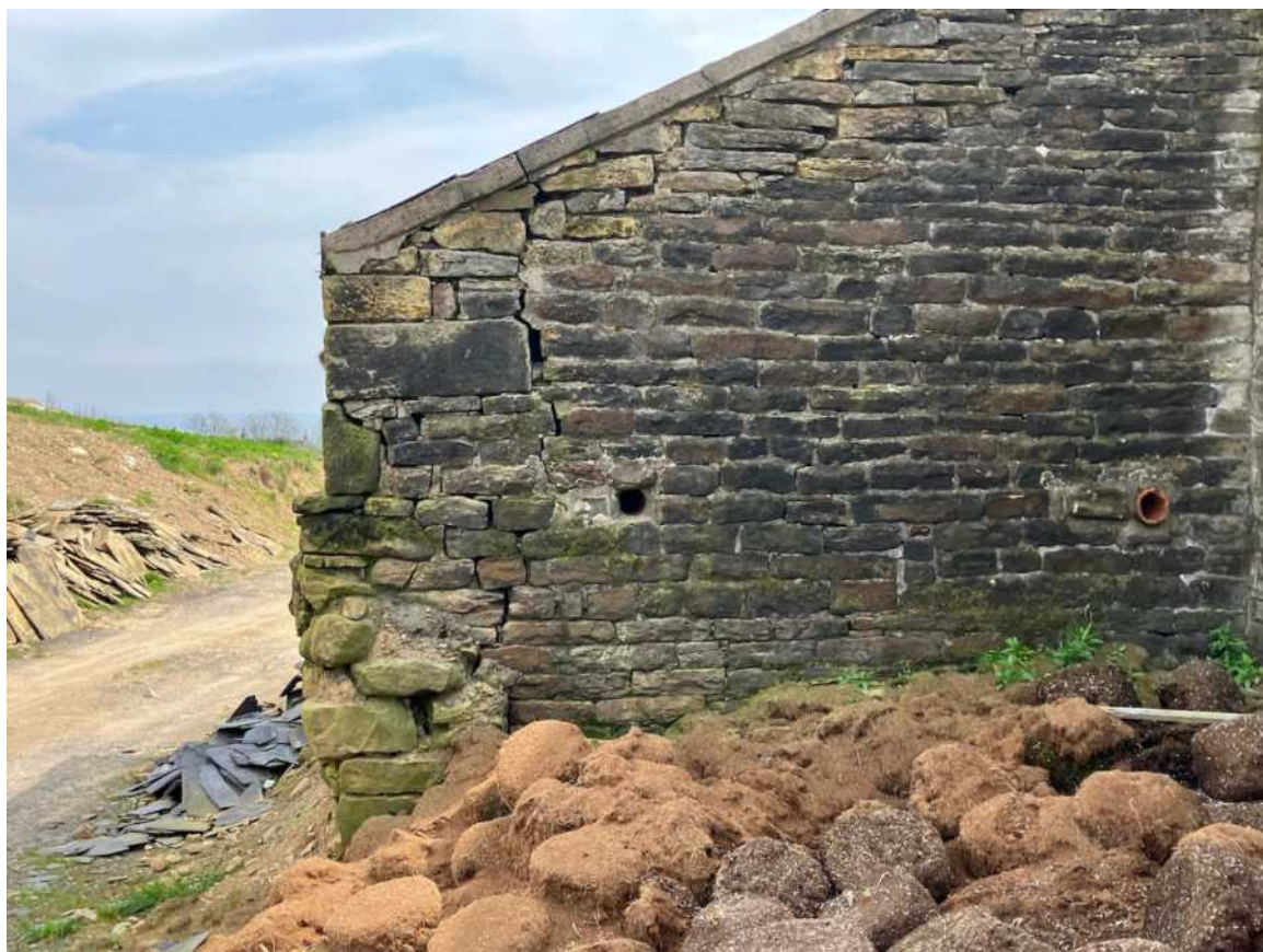
Photo 7: Lean-To Extension – Vertical Cracking
