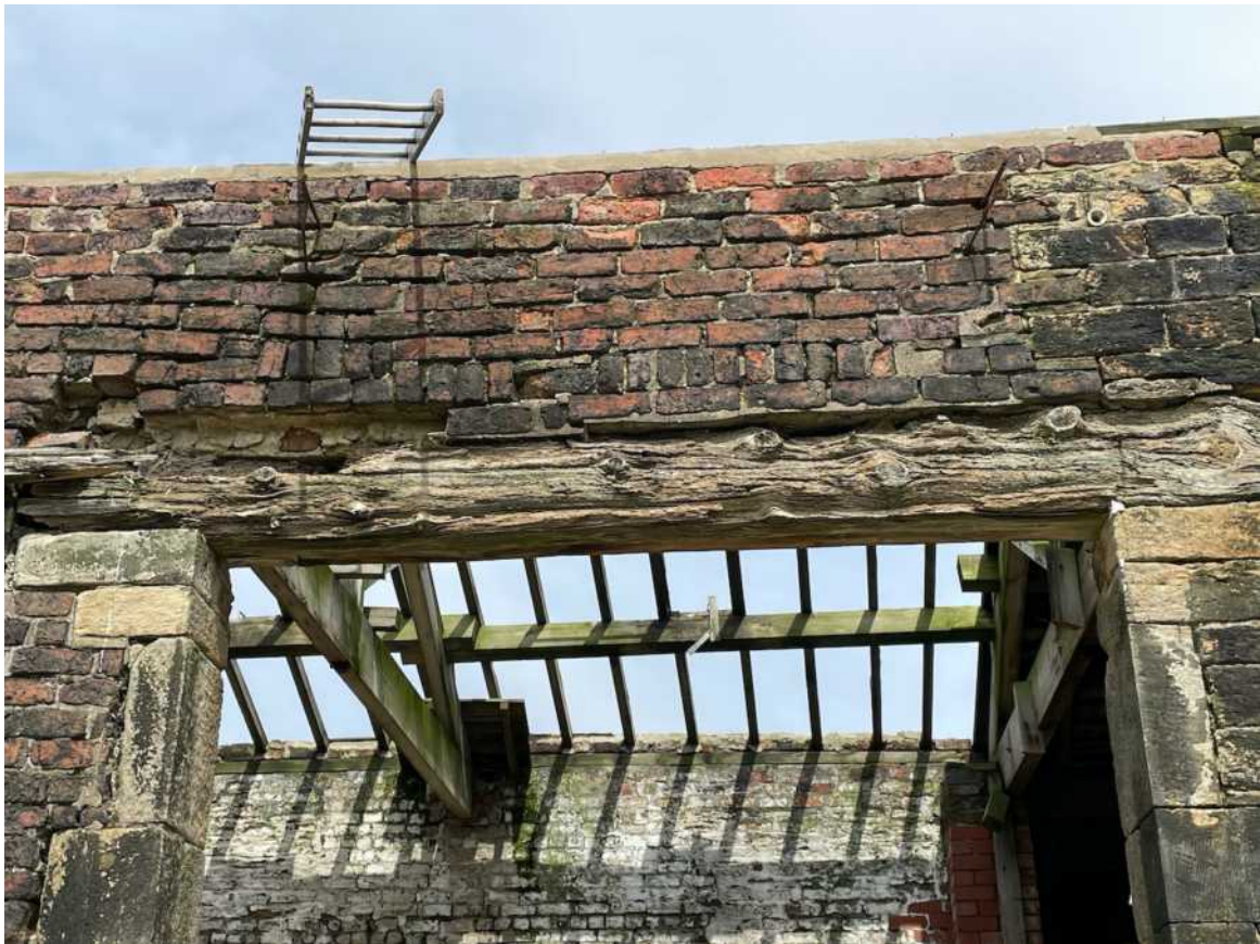
Photo 9: Cart Entrance - Decayed Lintel & Unconsolidated Masonry
