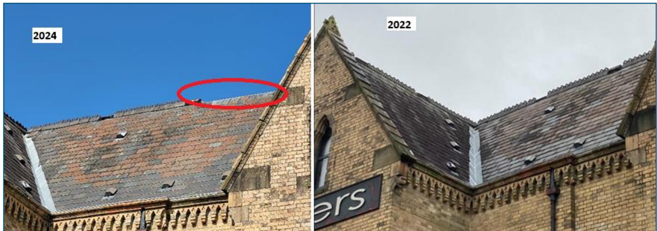
Photo 7: Showing section of missing ridge tiles in 2024 that were present in 2022.
