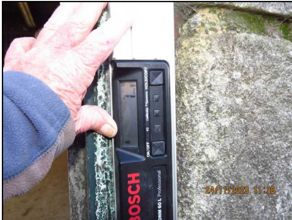
030 Good vertical alignment to right hand reveal
