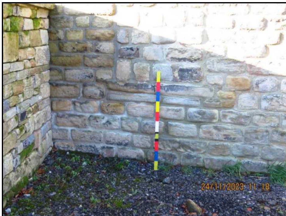
006 No signs of separation between wall structures
