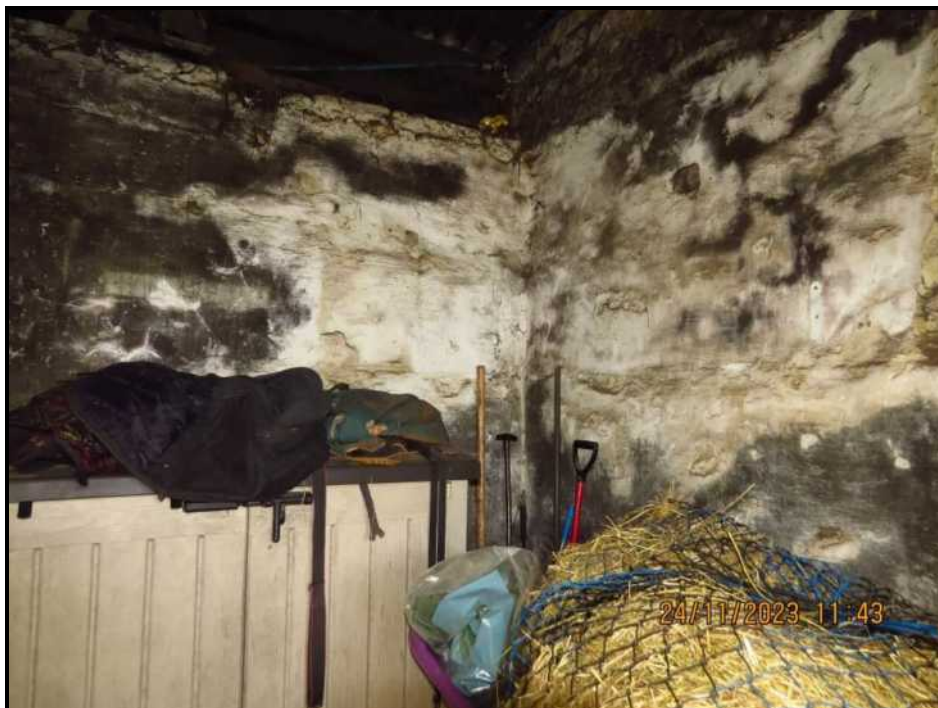
044 Lower wall, Northern corner
