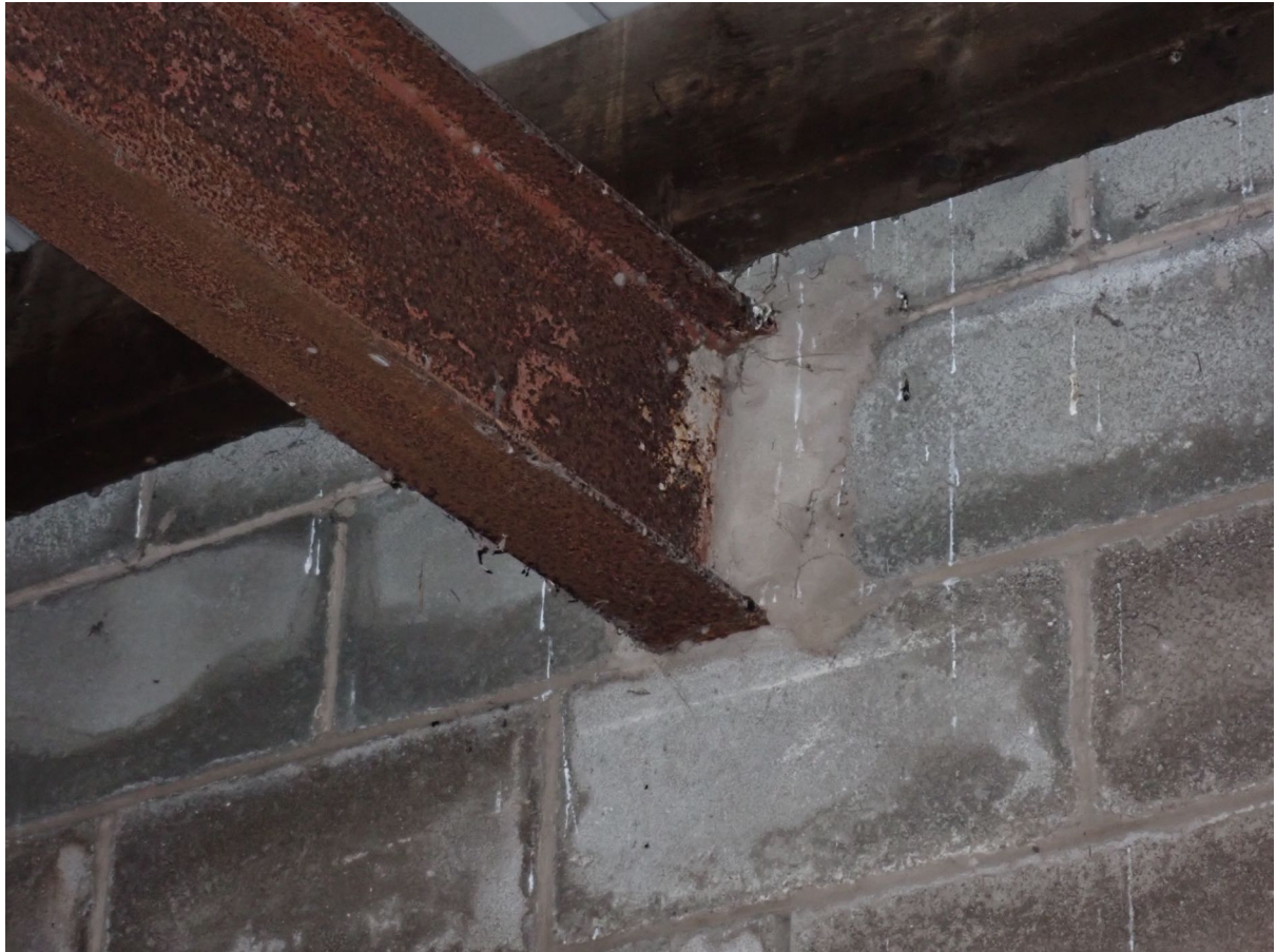
9 – Steels are fixed into walls with cement, with no suitable gaps between materials.
