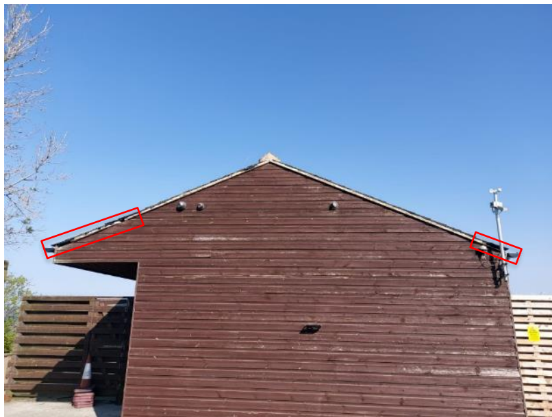
PLATE 12 SHOWING GAPS BETWEEN ROOF TILES AND WOODWORK
