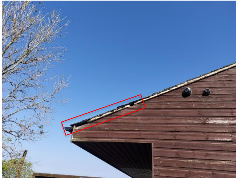
PLATE 13 SHOWING CLOSE UP OF GAPS BETWEEN ROOF TILES AND WOODWORK
