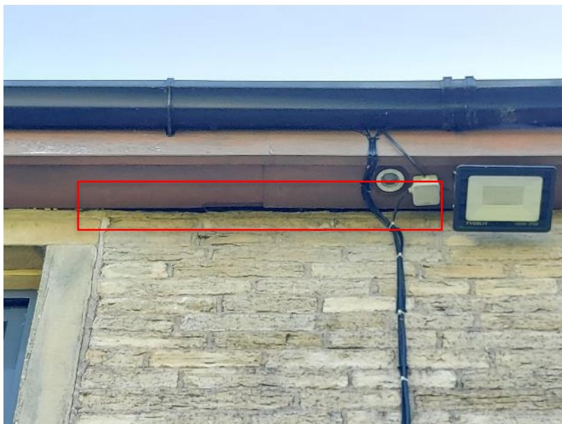
PLATE 6 SHOWING GAP BETWEEN BRICKWORK AND SOFFIT BOX
