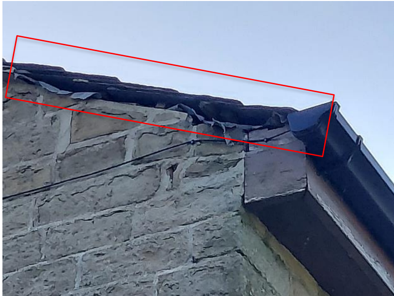
PLATE 5 SHOWING CLOSE UP OF GAPS ON NORTH WEST ASPECT
