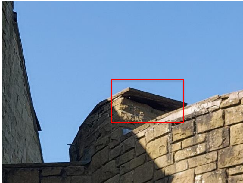
PLATE 8 SHOWING GAP BETWEEN ROOF TILE AND BRICK WORK
