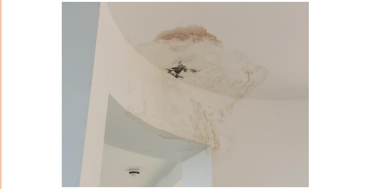
PLATE 10 SHOWING DAMP BELOW CHIMNEY
