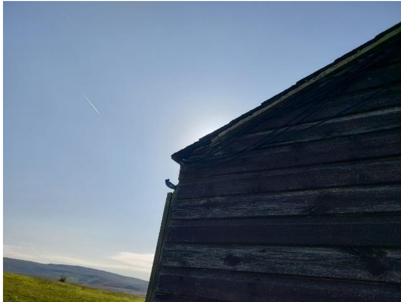
PLATE 15 SHOWING GAPS BETWEEN ROOF TILES AND WOODWORK
