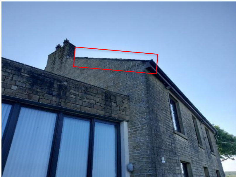
PLATE 4 SHOWING GAP BETWEEN ROOF TILES AND BRICKWORK ON NORTH WEST ASPECT
