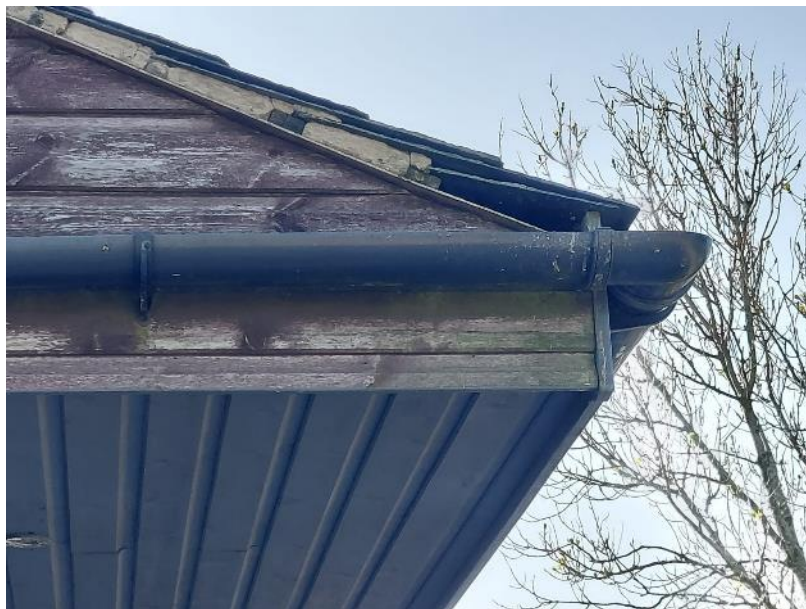
PLATE 16 SHOWING GAPS BETWEEN ROOF TILES AND WOODWORK
