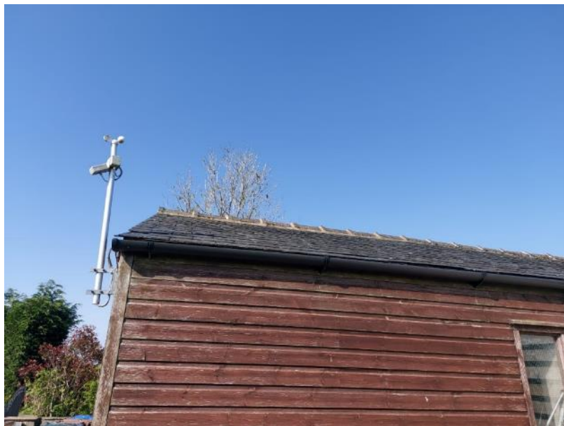
PLATE 14 SHOWING LIFTED TILES ON NORTH EAST FACING ASPECT
