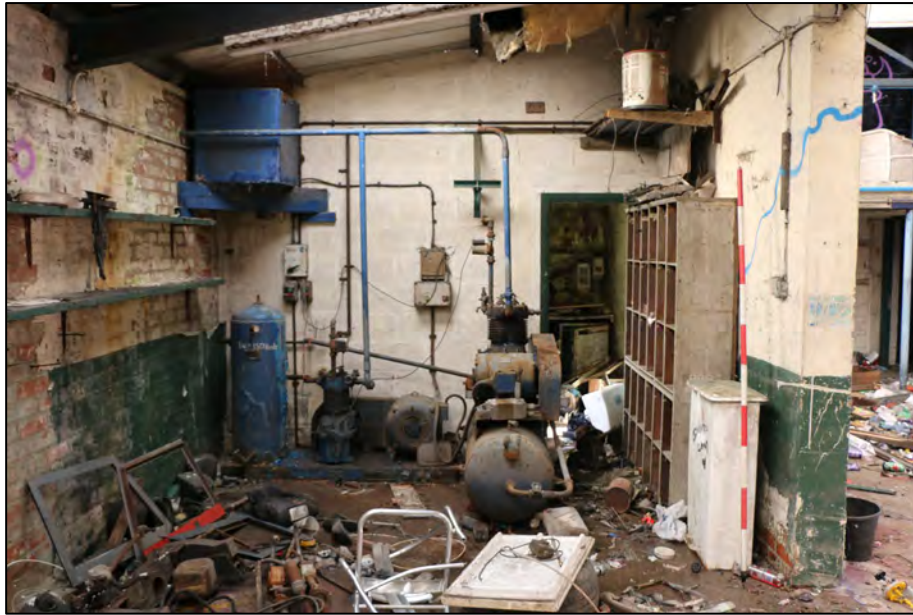
Photograph 19: Machinery in the eastern end of the northern room of Building 2, looking east.
