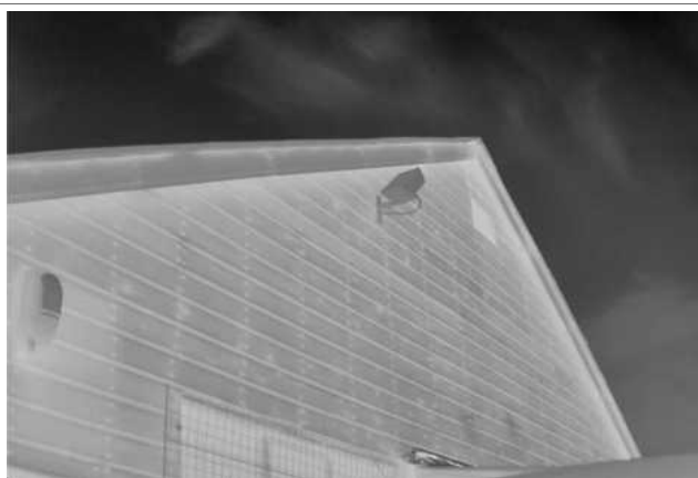
Thermal Camera Coverage
